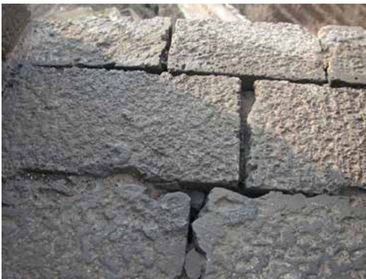
Picture 11. Gaps between the coating stones that comprise the dentils.
