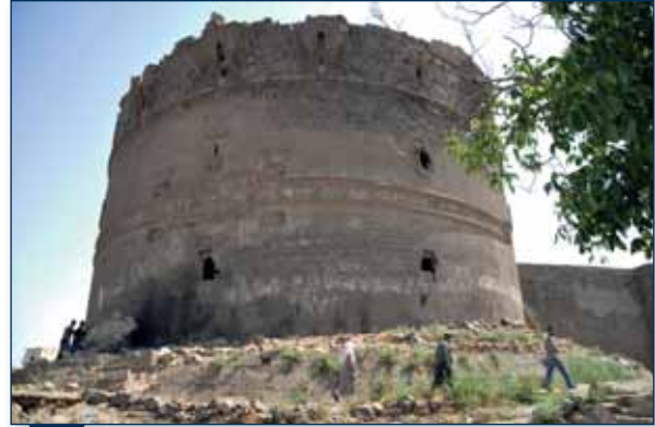
Image 4- 46: The traces on the tower arising from the fire near Ben U Sen Tower
