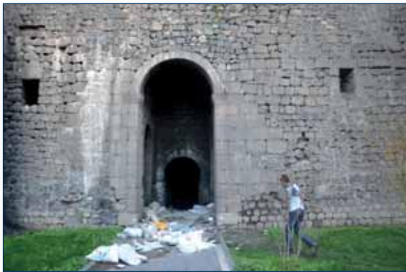
Image 4- 36 and Image 4- 37: The Towers are Used as a Garbage Dump because of being Disfunctional
