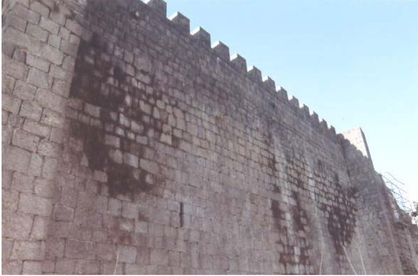
Picture 10. The humidity caused by the water flowing from the gargoyles and the deterioration in the stones.
