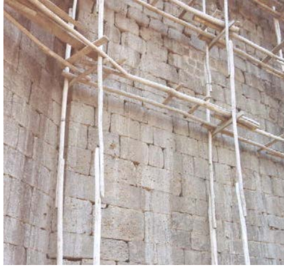
Picture 12. Attachment of the wooden scaffolds to the walls in a damaging manner.
