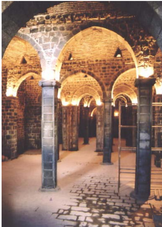
Picture 1. Wet floor boarding, the encircled columns and completely renewed column bases that are in contradiction with the authentic fabric.
