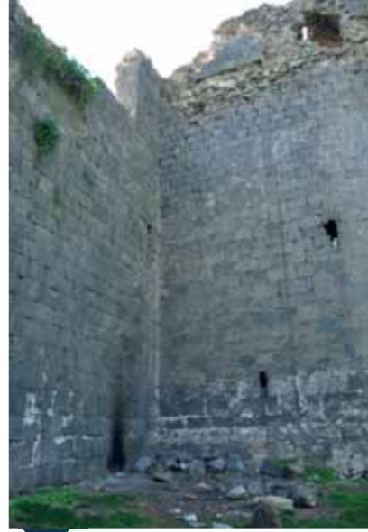
Image 4- 15: Stone Droppings on the North Side of the Tower number 16 (2013).
