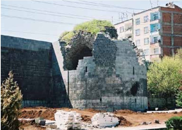
Picture 15. Wall façade that is covered with stone material that is not in harmony with the fabric.
