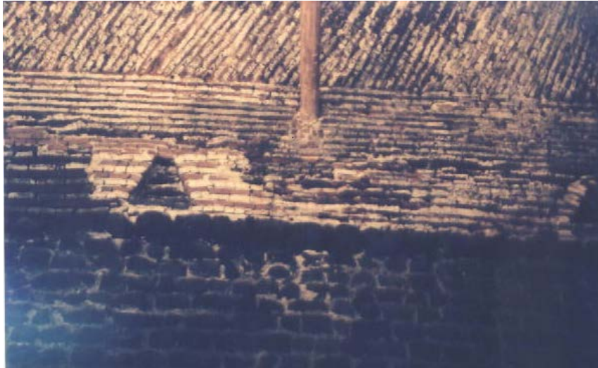
Picture 2 . Vaults that were painted to give the visual appearance of jointing.
