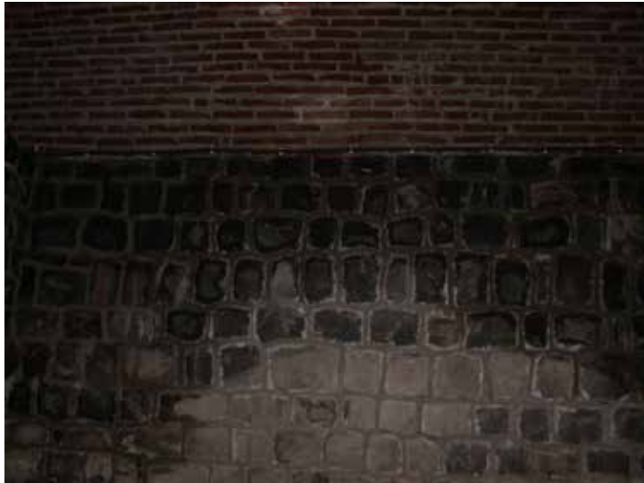
Picture 4. The damp surface formed on the wall due to unresolved insulation issues.
