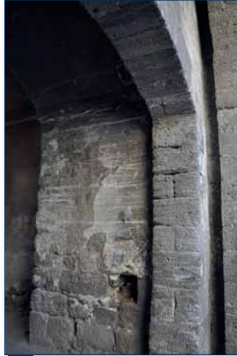
Image 4- 3: The destruction on Saray Gate caused by car passages
