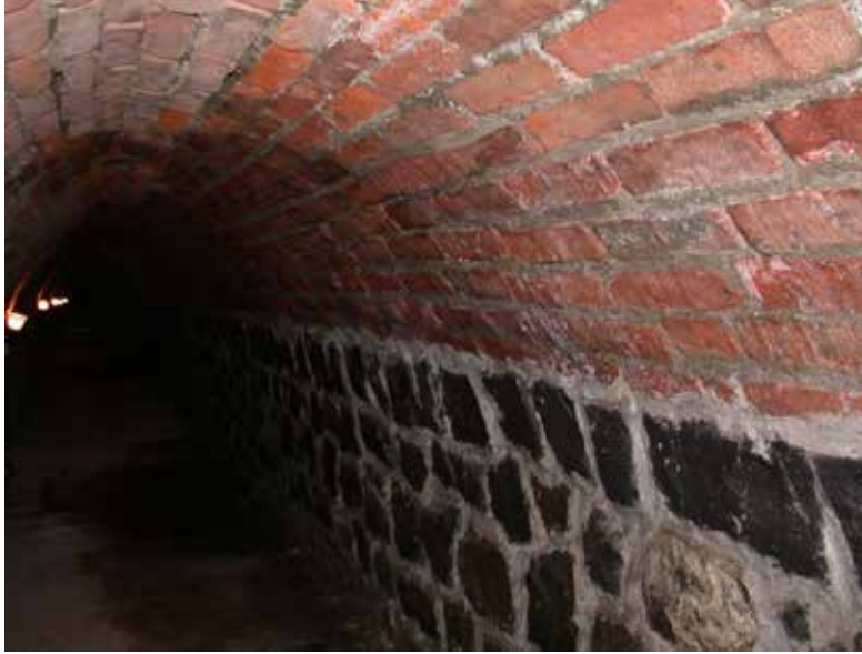
Picture 5. The humidity caused by the water flow from the terrace flooring due to lack of insulation.
