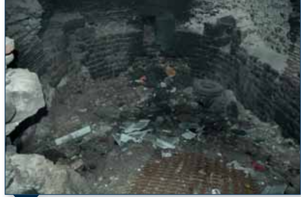
Image 4- 45: The deterioration arising from the fire inside of the towers and the wastes in the towers
