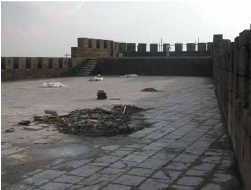
Picture 9. Tower's last section's status after the restoration (Which source was the plan based on and how it was completed and changed are unknown).
