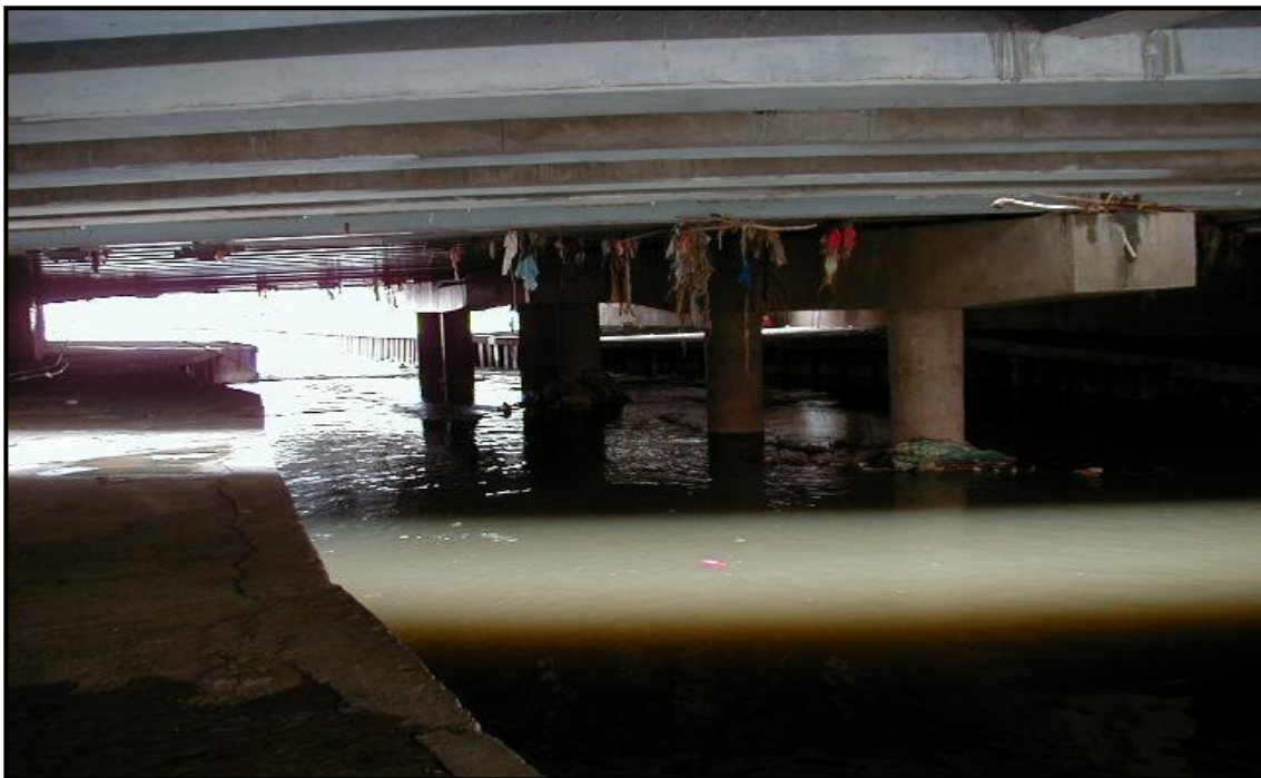
Figure C4: Klang River – Jln Tun Perak Bridge (view from left bank from upstream)
