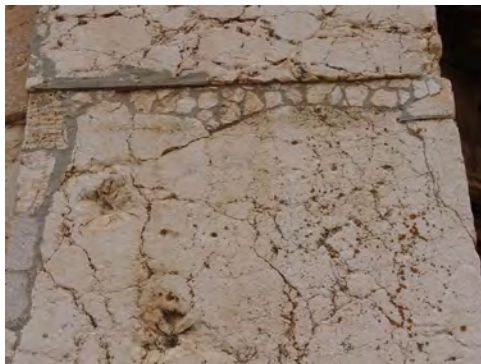
Figure 8.11: Star crack probably due to an internal iron peg from the interventions of the 60s
