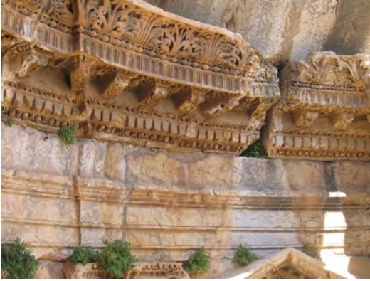
Figure 8.12: Entablature, the erosion due to rainwater leakage is visible
