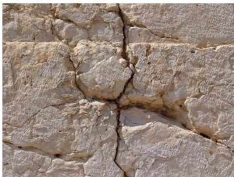
Figure 8.10: Restoration of a stone block with cement. The stone surface is already very highly fissured
