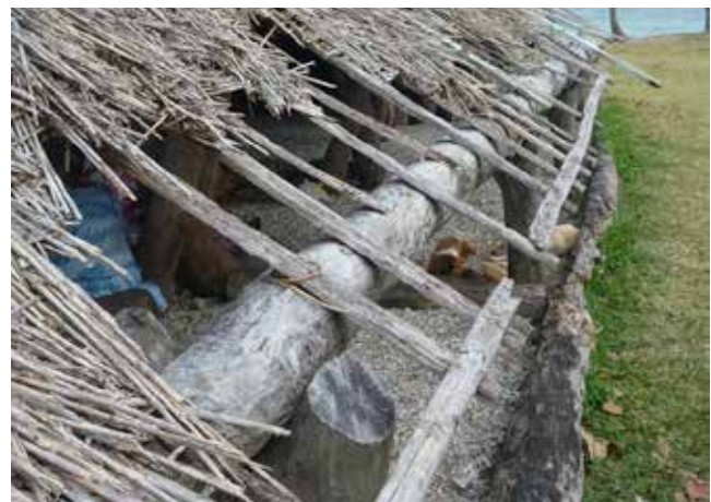
Figure 22: The damaged eaves over the side entry post- Tropical Cyclone Pam.
