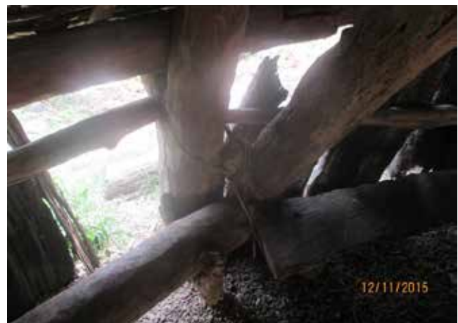
Figure 16: A break in the black palm wall might be evidence of damage made by Tropical Cyclone Pam.
