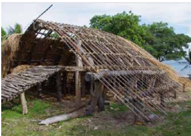
Figure 8: Photograph from 2010 showing the Taloa Farea under construction at a time when the wild cane thatching was being secured. Note the timber scaffolding near the front entry.
