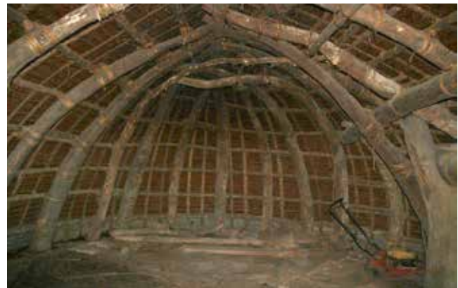
Figure 7: The curved structural posts form both the walls and the roof (pre- Tropical Cyclone Pam).
