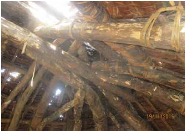
Figure 13: Image showing the complexity of the structural connections at the rounded end of the nakamal (post- Tropical Cyclone Pam).
