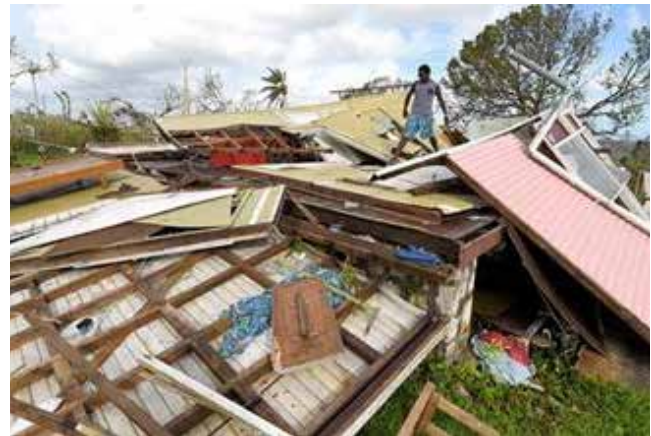
Figure 25: A house constructed from imported materials in Port Vila that was completely destroyed by Tropical Cyclone Pam.
