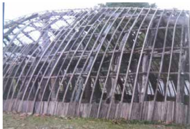
Figure 6: Photograph from 2010 revealing the structure of the farea during the rebuilding process.
