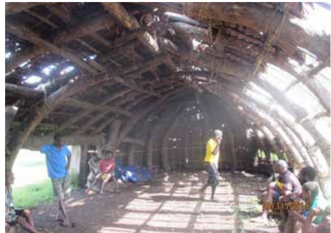
Figure 9: Post- Tropical Cyclone Pam, illustrating the interior of the nakamal and the damaged natangura roof.
