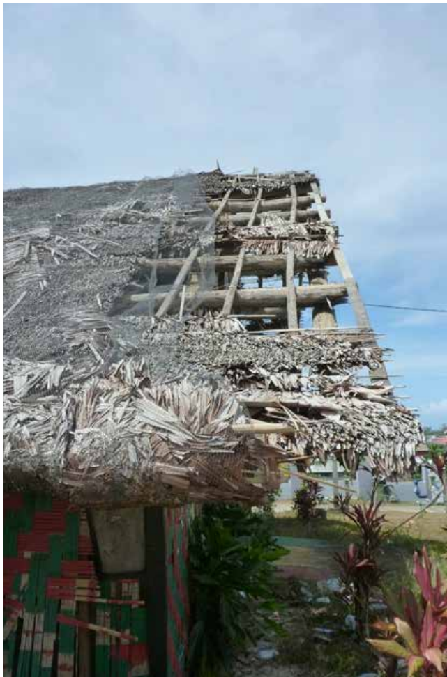
Figure 19: The damage caused by Tropical Cyclone Pam to the Chiefs' nakamal's roof thatching is particularly evident over the eaves.
