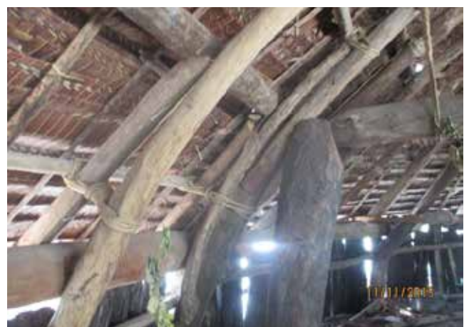
Figure 9: The interior roof structure post- Tropical Cyclone Pam.
