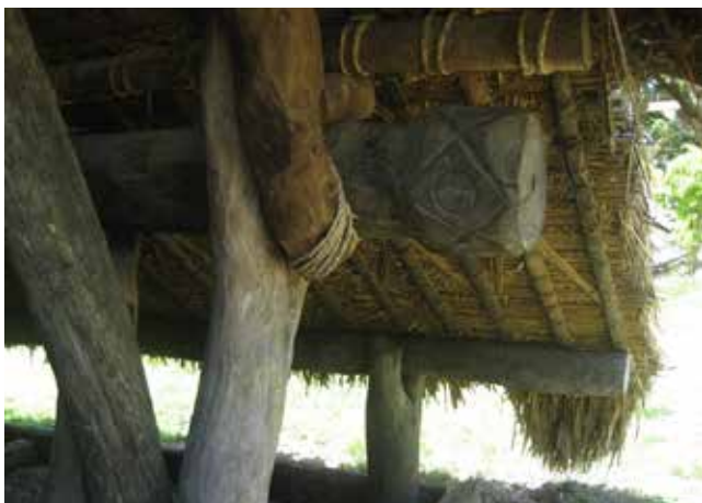
Figure 14: The carved edge beam at the front entry of the farea (pre-Tropical Cyclone Pam).
