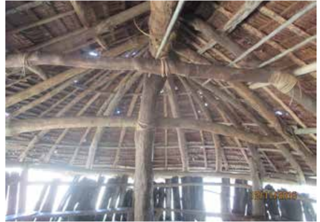
Figure 12: The rafters at both ends of the nakamal splay to fit the oval shaped plan (post- Tropical Cyclone Pam).
