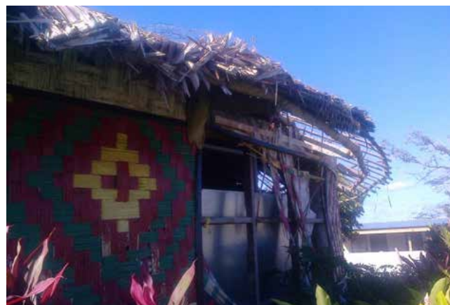
Figure 18: The rounded eaves and walls at the back of the Chiefs' Nakamal were damaged during Tropical Cyclone Pam.
