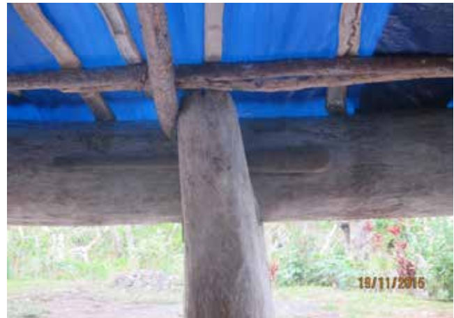
Figure 15: While the natangura roof was destroyed by Tropical Cyclone Pam, several structural members remain in tact.
