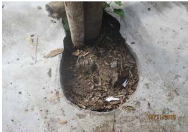
Figure 22: The damaged concrete slab post-Tropical Cyclone Pam showing where a post would have once been located.
