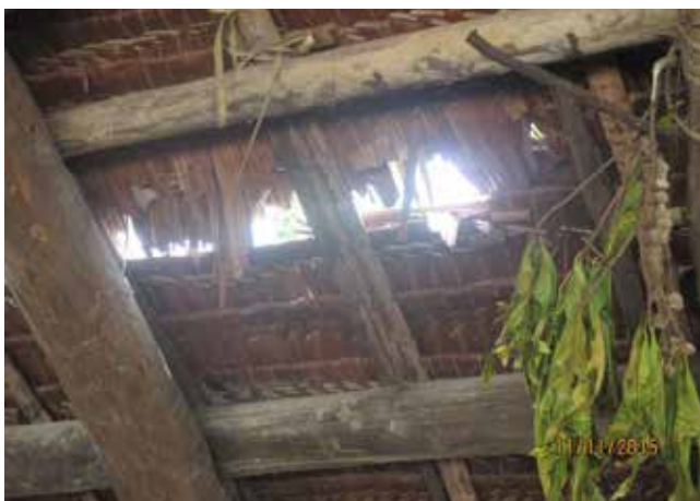
Figure 10: The roof of the nakamal was damaged by Tropical Cyclone Pam.
