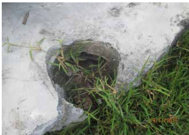
Figure 23: The damaged slab edge (post- Tropical Cyclone Pam).
