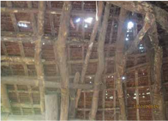
Figure 11: Holes were made in the natangura thatched roof during Tropical Cyclone Pam.
