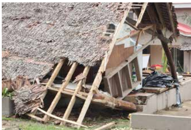
Figure 27: A house constructed from both traditional and imported materials that was completely destroyed by Tropical Cyclone Pam.
