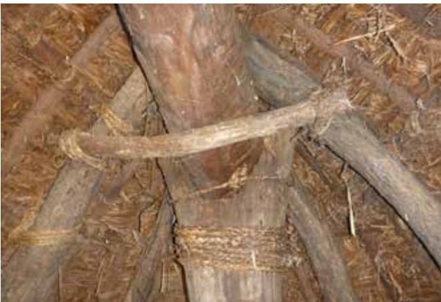
Figure 22: Roof connection detail on the Taloa Farea on Nguna Island, post-Tropical Cyclone Pam. The plaited pandanus rope connections remained intact despite the category 5 winds.
