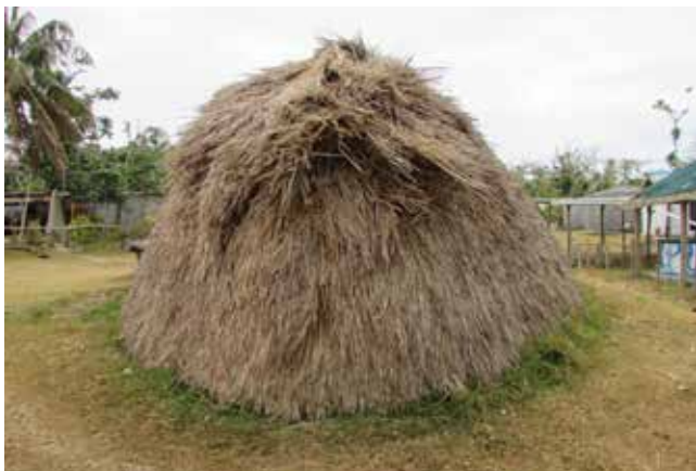
Figure 24: The back of the Taloa Farea on Nguna Island in October 2015, looking somewhat ruffled after Tropical Cyclone Pam.
