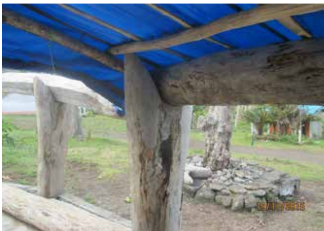
Figure 14: A blue tarpaulin is fixed to the roof battens in place of the natangura roof thatching. All of the roof thatching on the Mangarisu Nakamal was destroyed by Tropical Cyclone Pam.
