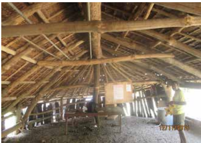
Figure 8: The interior of the Moriu Nakamal (post- Tropical Cyclone Pam), illustrating the structural system made from local hardwood.
