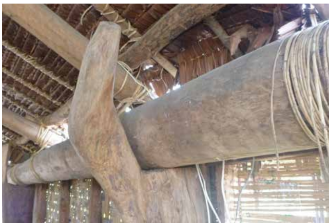
Figure 25: Column/post detail post- Tropical Cyclone Pam. While the structural members remained significantly in tact, the rope tie-down details show signs of damage.
