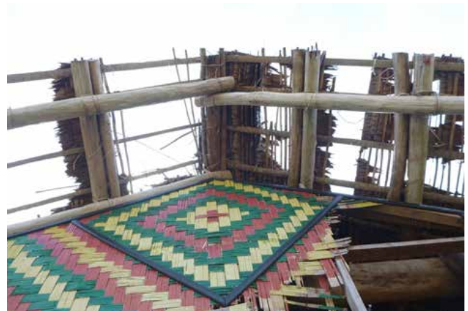
Figure 20: The damaged roof and wall thatching at the front of the Chiefs' Nakamal post- Tropical Cyclone Pam.
