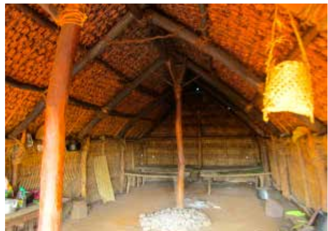
Figure 9: Interior view of the Erromango Nakamal post- Tropical Cyclone Pam.
