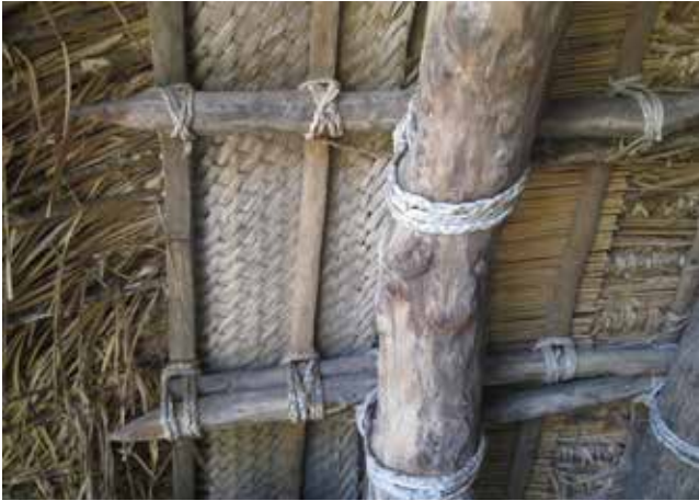
Figure 17: The layers of texture at the roof edge, including woven pandanus, chamfered battens and wild cane thatching (pre- Tropical Cyclone Pam).
