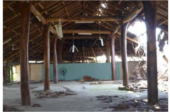
Figure 23: While the main structure remained intact during Tropical Cyclone Pam, the secondary structural members and traditional cladding/roofing materials were damaged by the high winds.
