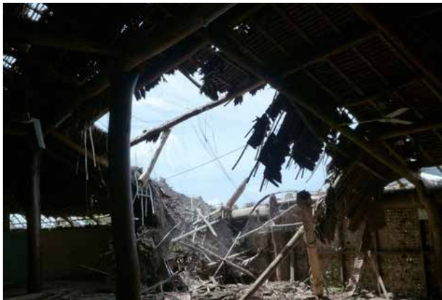
Figure 24: Image showing the hole made in the roof to the Chiefs' Nakamal by Tropical Cyclone Pam.
