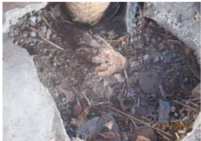
Figure 21: The damaged concrete slab (post-Tropical Cyclone Pam).
