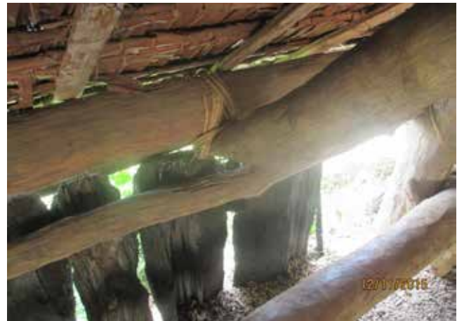
Figure 15: Roof/wall junction of the Moriu Nakamal (post- Tropical Cyclone Pam).
