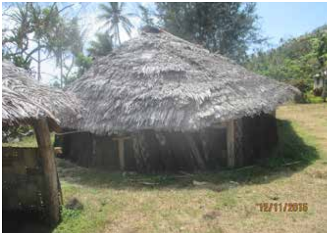
Figure 7: This picture suggests that some of the black palms trunks that infill the walls were weakened by Tropical Cyclone Pam.
