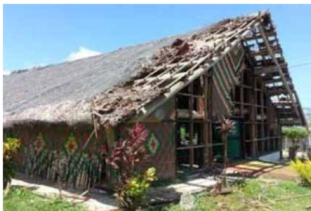
Figure 17: The damage caused by Tropical Cyclone Pam to the front eaves of the Chiefs' Nakamal.
