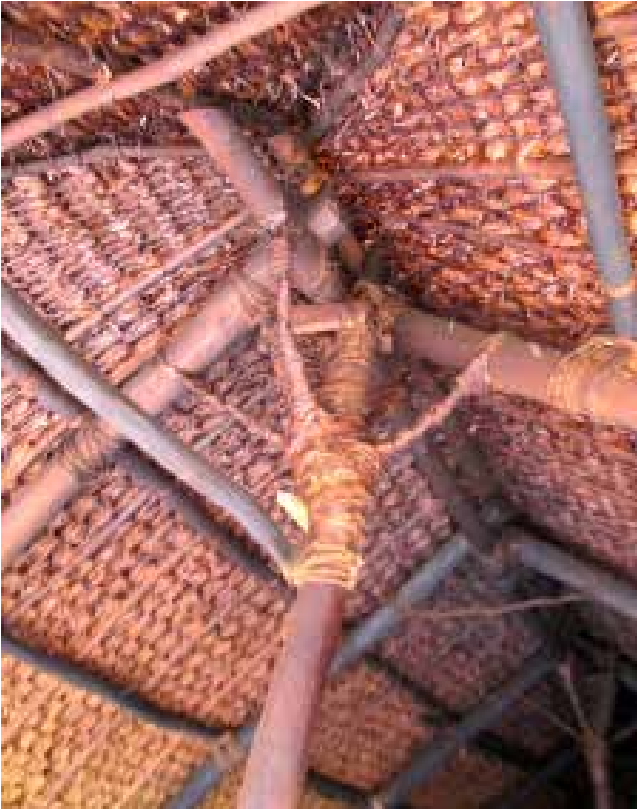
Figure 10: The underside of the roof thatching on the Erromango Nakamal (post- Tropical Cyclone Pam). Note that the natangura has remained in good shape.
