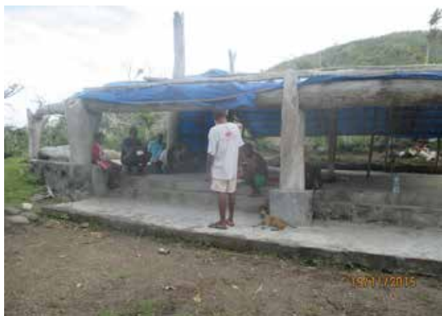
Figure 11: A tarpaulin covers the damaged roof of the Mangarisu Nakamal post- Tropical Cyclone Pam.
