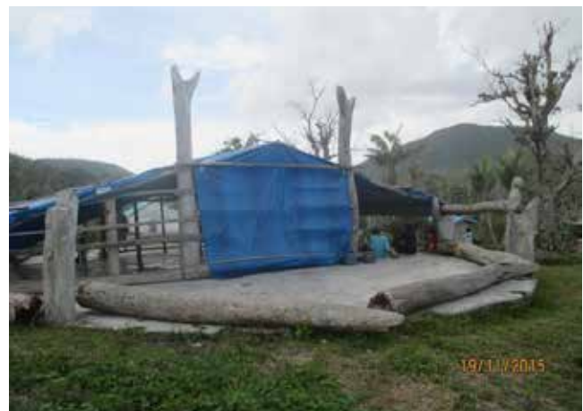
Figure 10: What remains of the Mangarisu Nakamal post- Tropical Cyclone Pam. Note that the structural members to the end bay have been completely destroyed.
