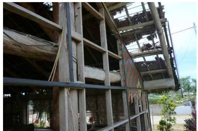
Figure 21: Tropical Cyclone Pam stripped the front elevation of the Chiefs' Nakamal of its wall cladding and significantly damaged the natangura roof thatching.
