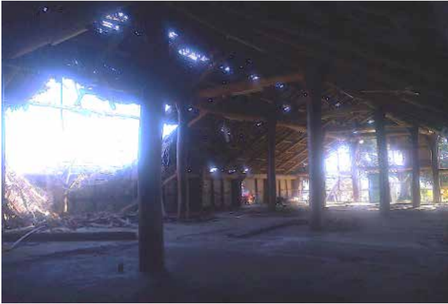
Figure 22: The interior of the Chiefs' Nakamal post- Tropical Cyclone Pam. A significant hole was torn in the roof over the centre of the nakamal.
