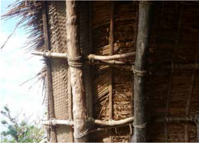
Figure 23: The damaged eave over the front entry post- Tropical Cyclone Pam.
