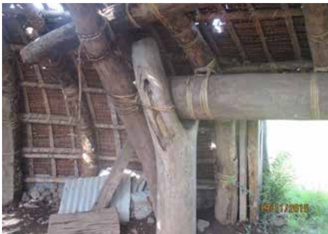
Figure 14: The large structural members at a post / beam junction (post- Tropical Cyclone Pam).
