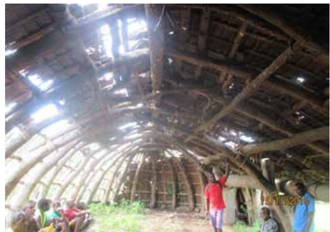
Figure 10: The interior of the nakamal and the damaged natangura roof post- Tropical Cyclone Pam. Note the weeds growing though the earth floor
