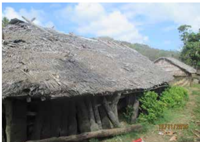
Figure 5: The exterior walls of the Moriu Nakamal, which are made from black palm trunks (post- Tropical Cyclone Pam).
