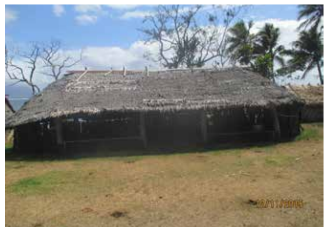
Figure 4: The Moriu Nakamal on Epi Island (post- Tropical Cyclone Pam) sustained minimal damage from the cyclone.
