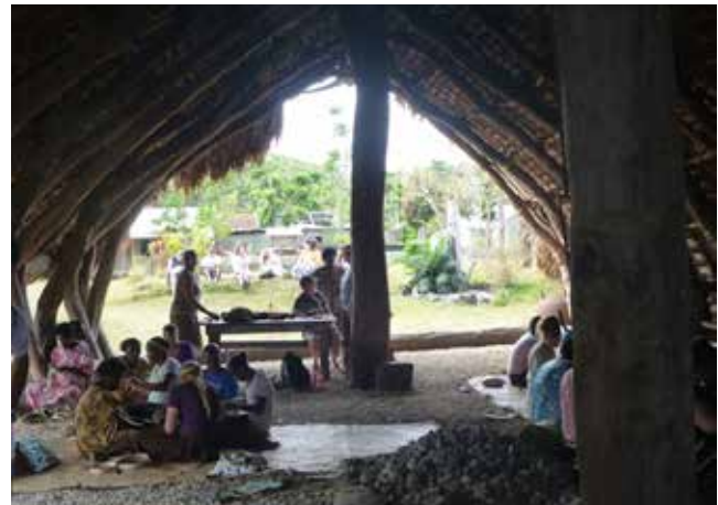
Figure 21: View from inside the farea looking back towards the front entry, showing how the farea could still be used despite the damage caused by Tropical Cyclone Pam.
