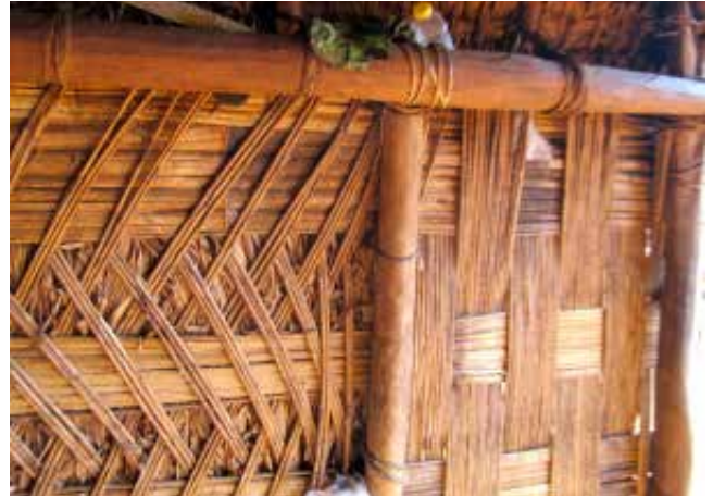
Figure 11: The wall cladding to the interior of the Erromango Nakamal (post- Tropical Cyclone Pam), which has remained in good condition.
