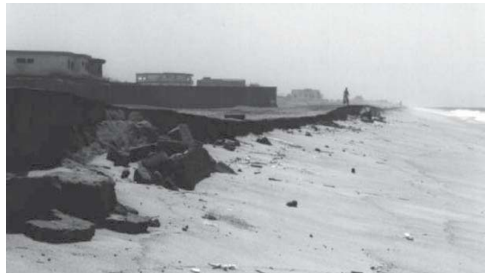
Beach Erosion in Cotonou and related road destruction
