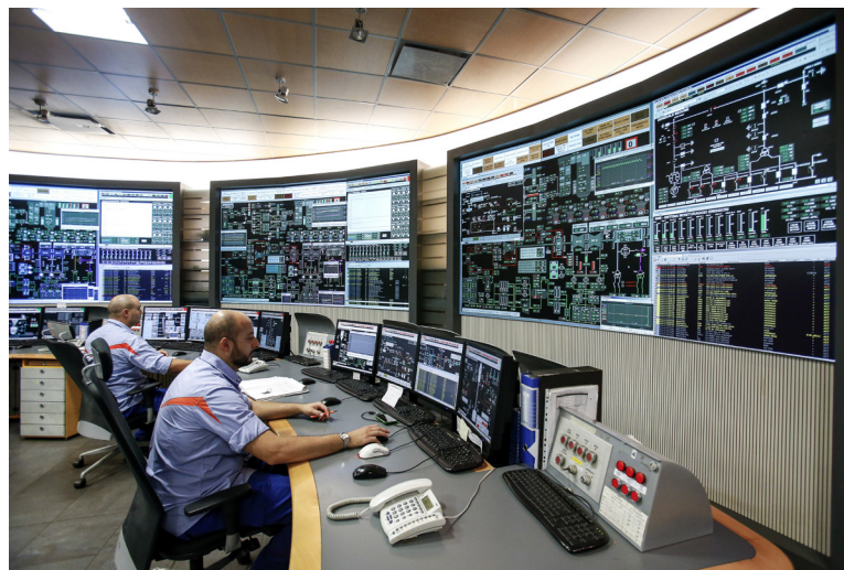
Employees monitoring operational data in Civitavecchia (Italy) Photo: © Alessia Pierdomenico/Shutterstock.com
