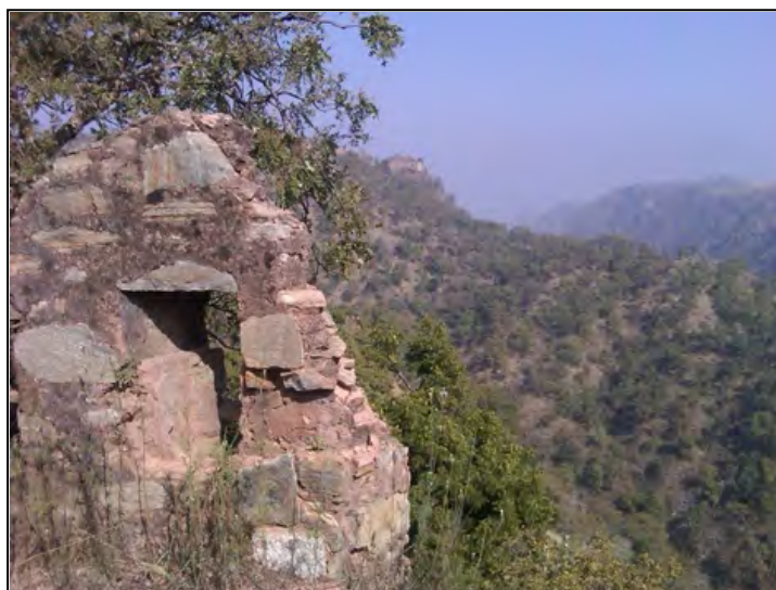
A fortification battlement in a ruinous condition- a common feature among the fort walls extending into the forests
