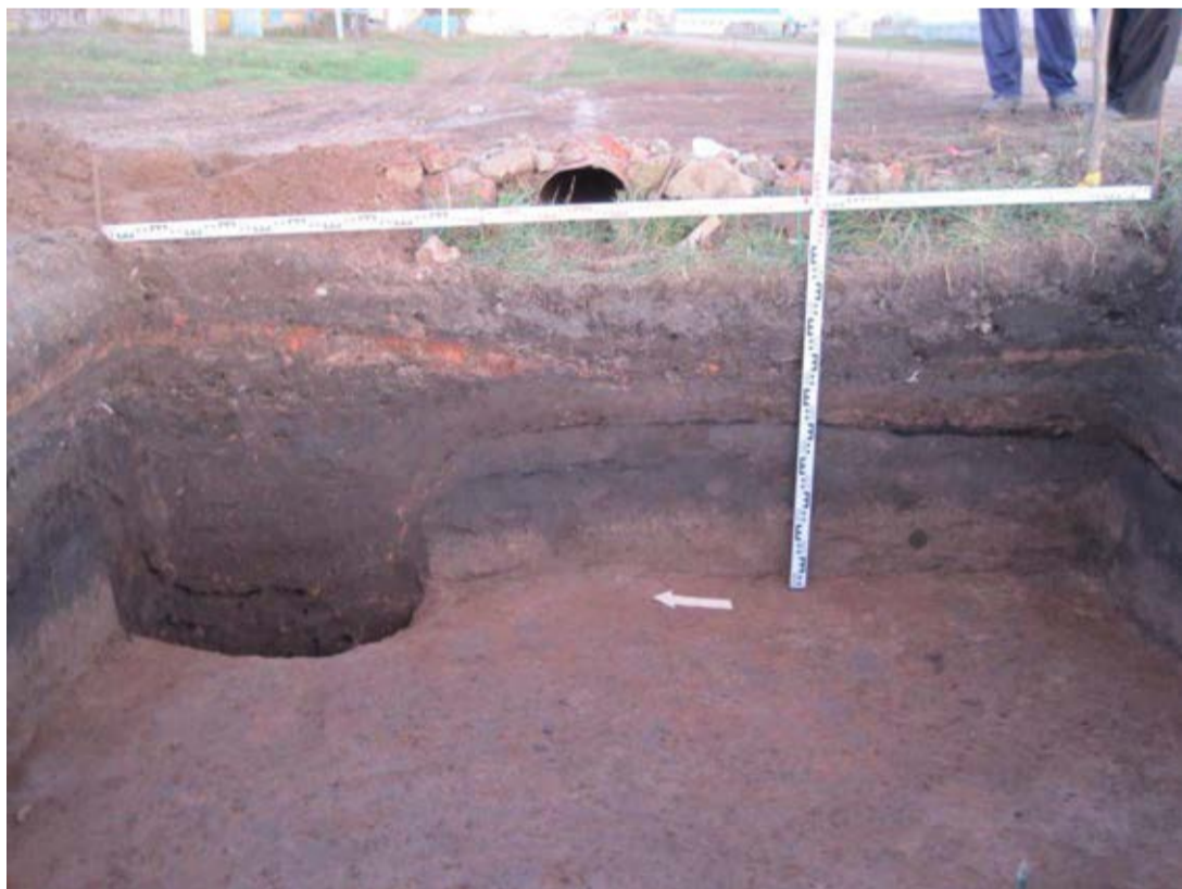
Water conduit. Pit-hole No.4 on Nazarovy Str. near the river boat station
