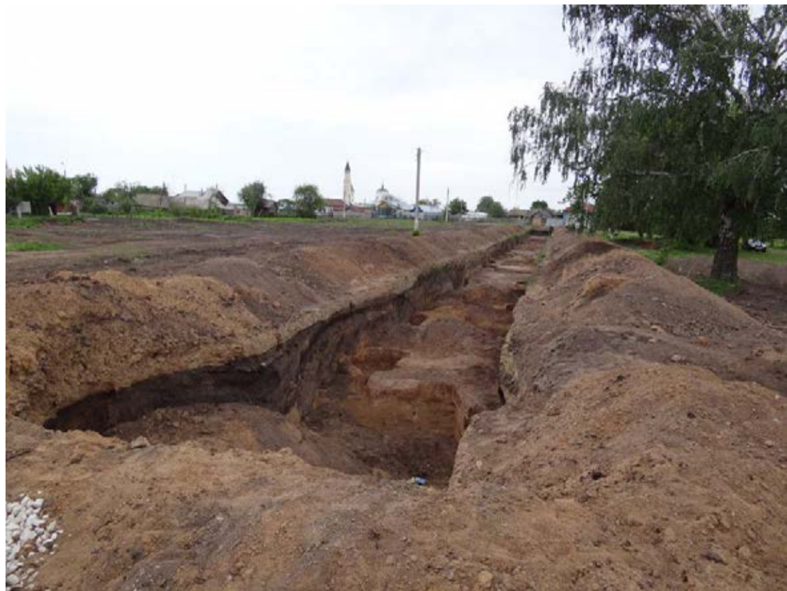
General view of CLXXVIII excavation on the spot of road construction towards the car park.
