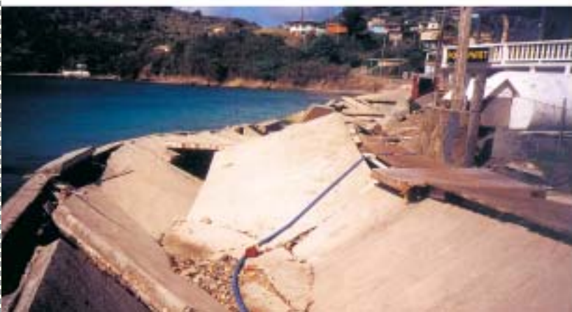
Hurricane Lenny caused serious damage to the coastal road at Hamilton, Bequia in 1999
