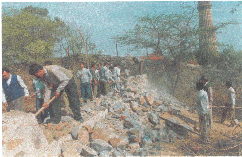
ENCROACHMENTS, ILLEGAL CONSTRUCTIONS IN THE BUFFER ZONE
