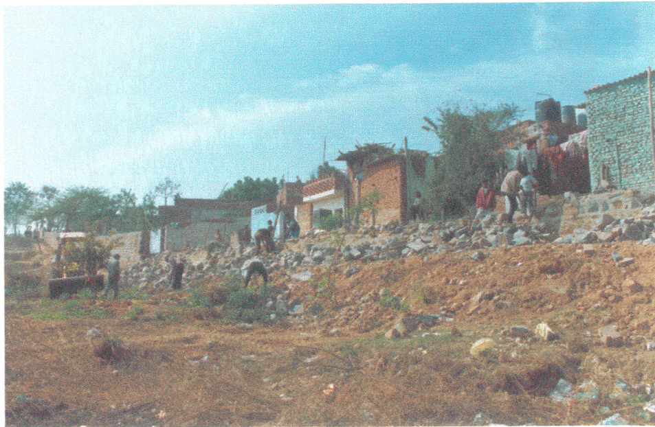
ENCROACHMENTS, ILLEGAL CONSTRUCTIONS IN THE BUFFER ZONE
