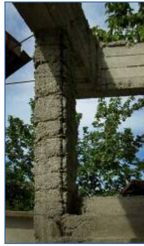
Fig. 7 LEFT: House being reconstructed to replace one destroyed in Afyon earthquake. Concrete is being mixed on ground with garden hose and without slump test or measurements.
