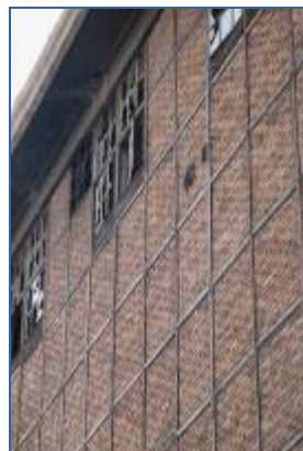
Fig. 33 Detail of masonry wall in Istanbul's Silahtarağa Powerplant showing brick infill with horizontal and vertical light-frame steel "I" sections. (Kıraç et al, 2003) This construction is similar to that shown in Figure 35 below.
