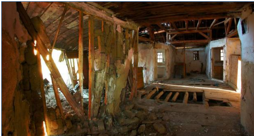
Fig. 64 This house in Elden had been abandoned for years before the earthquake. Despite its deteriorated condition, the earthquake damage was limited to the collapse of some of its walls. The basic rough construction characteristic of a rural area without a saw mill or access to a kiln can be seen with the undressed logs used for the structure, and unfired adobe blocks used for the infill.
