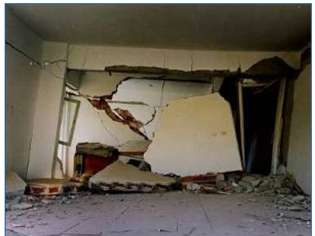
Figure 36: Collapse of a brittle interior hollow clay block wall illustrating typical failure pattern for such walls lacking subdivisions.
