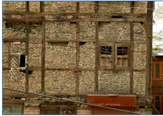
Fig. 15 Example of Dhajji Dewari construction in Srinagar, 2005. The timbers form a complete frame, and the masonry is inset into the frame.
