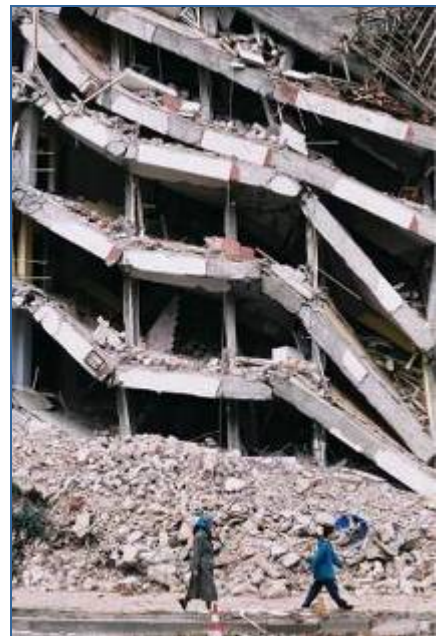
Fig. 20 Partial collapse of RC Building, Gölcük , Turkey, 1999.
