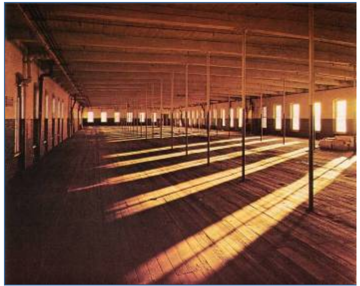
Fig. 11 Interior of an 1840 Amoskeag mill building constructed with heavy timber floors, iron columns, and brick exterior walls connected to the floors with iron anchors.
