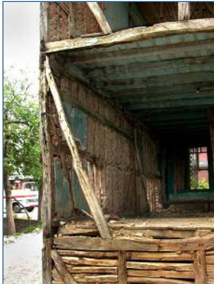
Fig. 40 Partially demolished house in Golcuk showing the single brick wythe thickness of typical himiş wall. On the LEFT is the exterior and on the RIGHT is the interior face of the same wall.
