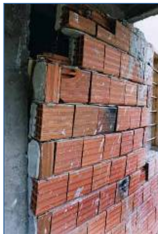
Fig. 25: Infill wall RC building in Mexico City damaged in 1985 earthquake. The infill masonry in this structure almost caused the collapse of the building. The damage to the corner column that left the building teetering on the edge of collapse can be seen on the right.
