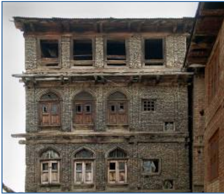
Fig. 14 Example of Taq construction in Srinagar, Kashmir, 2005. The timbers in the masonry walls only run horizontally parallel to the wall and through the wall.
