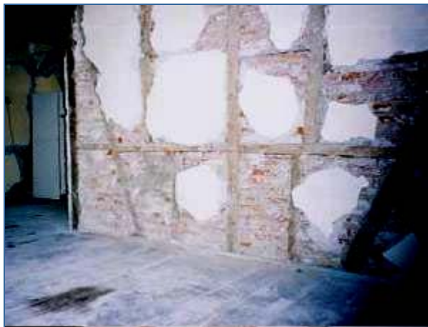
Figure 35: Hımış interior wall in house in Düzce earthquake damage district showing "working" of wall that caused loss of plaster.
