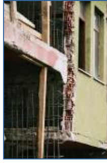
Fig. 28 & 29: Five story building damaged in the 1999 Düzce earthquake in Turkey, being retrofitted with reinforced concrete shearwalls. No.30 shows the existing hollow clay block walls removed and steel being inserted for the construction of a reinforced concrete shearwall. These images illustrate the extent of the work, and disruption needed for earthquake strengthening using shearwalls. The occupants had to move out for the duration of this work as many existing walls were removed.
