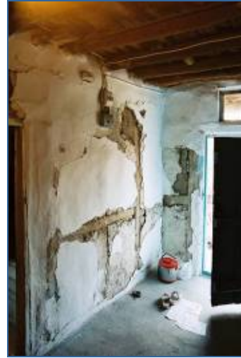
Fig. 46 Interior vestibule of house in Adapazari after the 1999 Izmit earthquake.
