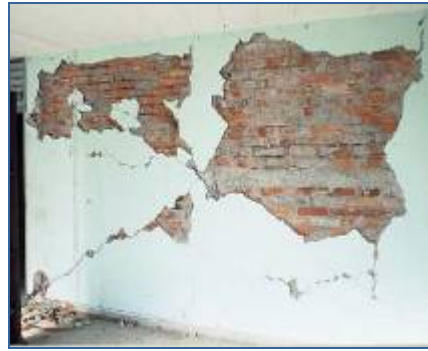
Fig. 31 Infill RC building in Mexico City after the 1986 earthquake collapsed many buildings nearby, including the one in Figure 20. Each infill wall is subdivided vertically and horizontally into 4 panels. Fig. 32 A subdivided internal brick infill wall in San Salvador after the 1986 earthquake.
