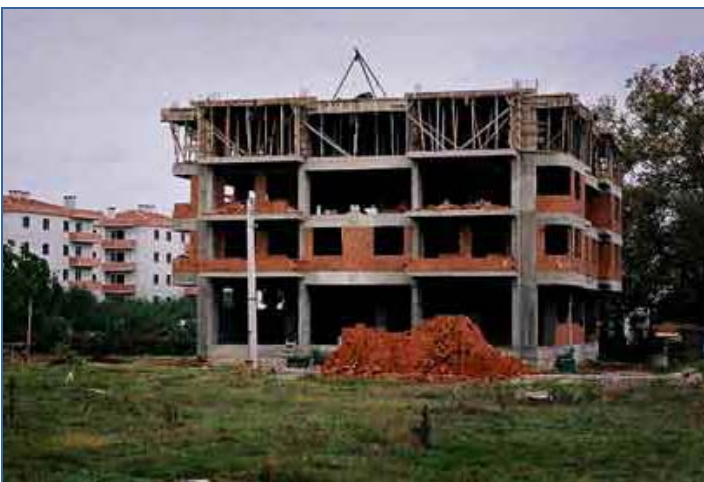
Fig. 21 Typical Turkish RC building under construction showing the hollow block infill being installed.
