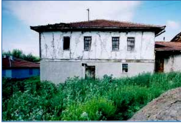
Fig. 44 LEFT: House in Orta, Turkey one day after the 2000 Orta earthquake – showing plaster cracking that reveals the timber frame. There was no evidence of damage beyond that of the cracked plaster.
