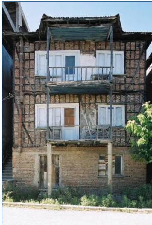
Fig. 9: This three story house in Gölcük located less than one km from the fault was undamaged by the 1999 earthquake, while a number of reinforced concrete buildings on the adjacent blocks collapsed. 1
