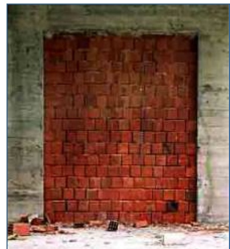
Fig. 22 Typical hollow clay block infill as used in reinforced concrete residential construction in Turkey.
