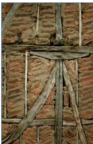
Fig. 1 Detail of traditional hımsı construction in Turkey in mid-20th century house in Gölcük.
