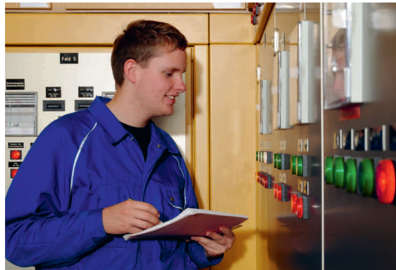
Process control in a water supply plant, Germany 2010
