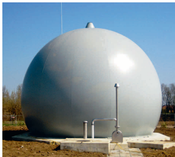
Gas Storage Tank from Wastewater Treatment Plant, Croatia 2012
