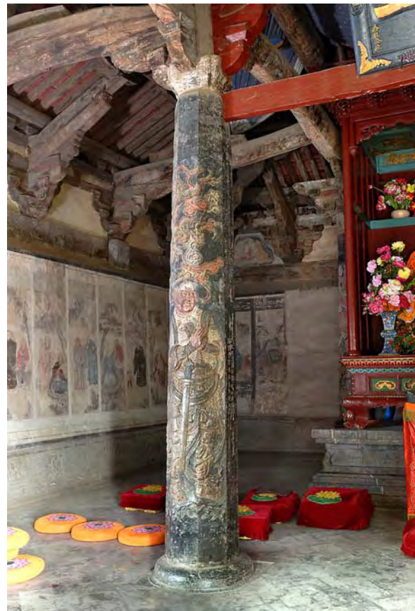
Photograph-5-34 Spar frame within Main Hall of Chuzu Temple of Shaolin Temple
