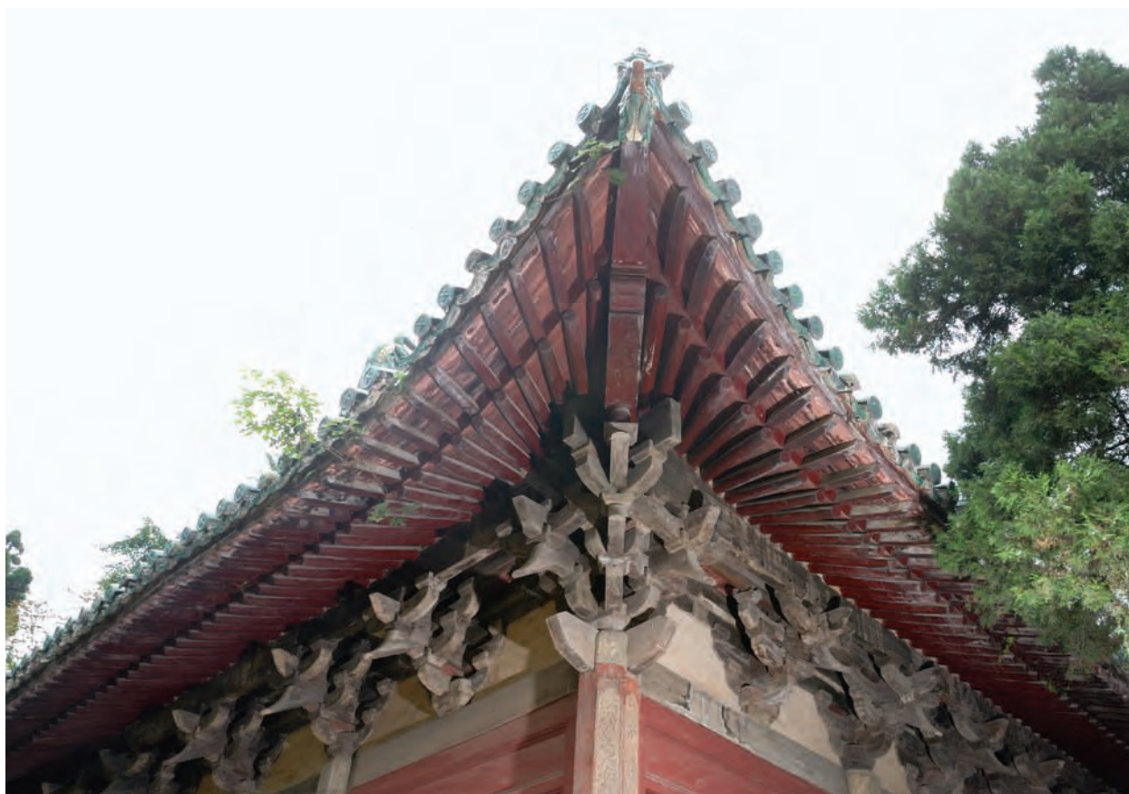
Photograph-5-30 South-western corner of the Main Hall of Chuzu Temple of Shaolin Temple
