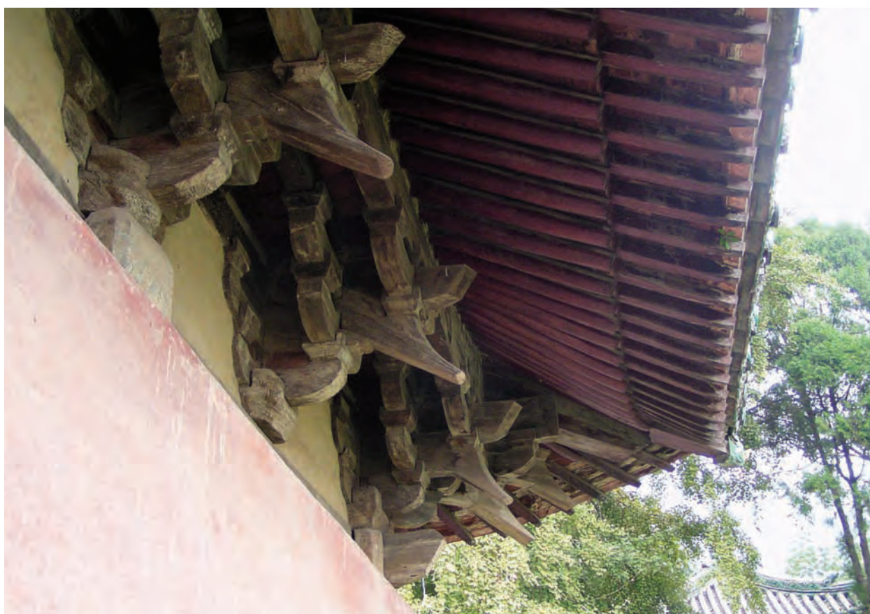
Photograph-5-31 Bracket set on Main Hall of Chuzu Temple of Shaolin Temple ( I )
