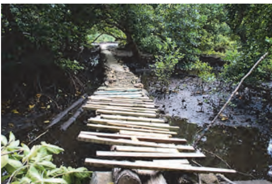
Photo 32 Accumulation of silt near a land bridge
