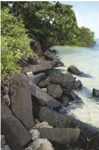
Photo 29 Collapse of the stonewall and the sedimentation of sand
