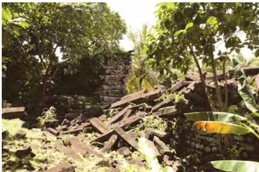
Figure 4.6. Collapse of the north perimeter wall seen from inside, Nandowas Islet (#113) (Kataoka et al. 2012:20, Photo 17).
