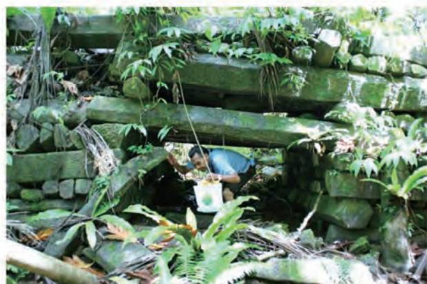
Photo 4 Ground subsidence around the entrance in the northwest outer wall
