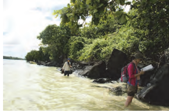
Photo 28 Collapse of the stonewall and the sedimentation of sand
