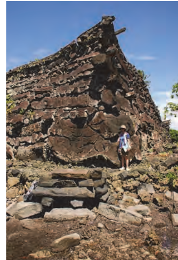
Photo 18 Crack in the massive basalt boulder in the southeast corner of the outer wall
