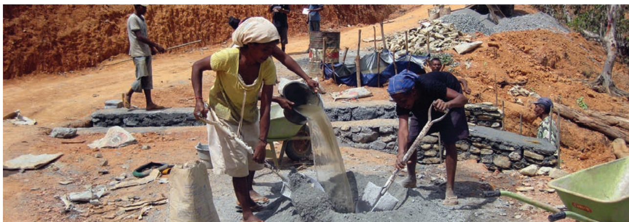
Rehabilitation of rural roads using labour-based techniques, through the ILO/ERA (enhancing rural access) project, funded by the European Union.
