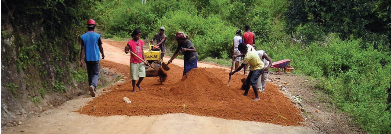
Rehabilitation of rural roads using labour-based techniques, through the ILO/ERA (Enhancing Rural Access) project, funded by the European Union.
