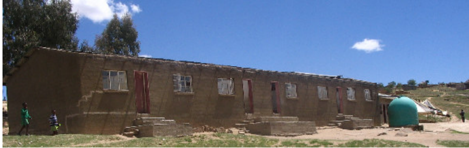
Motati Primary School in Leribe: Lower-cost, community-built school roof blown off
