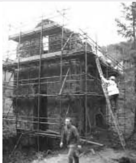
The Riverside Engine House at Gunnislake Clitters Mine within the Tamar Valley. The high quality restoration of the Riverside Engine House won a prestigious award for preservation from the Cornish Buildings Group in 2001. The Riverside Engine House during restoration.
