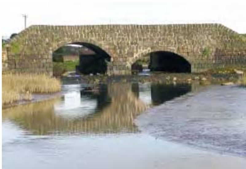
Black Road embankment and Black Bridge (1811, Scheduled Monument). The extensive use of scoria blocks is apparent.
