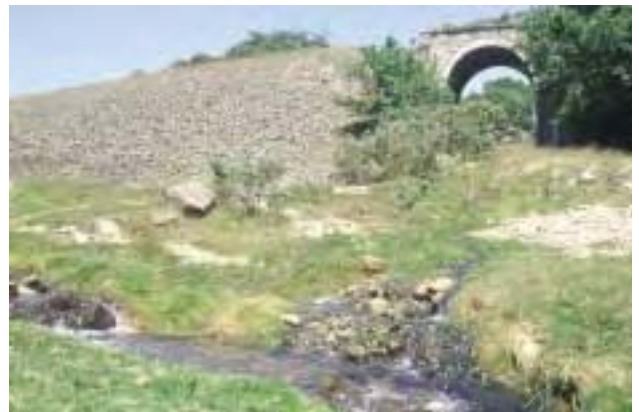
Liskeard and Caradon Railway bridge (Listed Grade II) and embankment at South Caradon Mine. The Seaton Stream in foreground.
