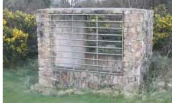
Mine shaft safety enclosure at Tresavean Mine, Lanner, designed to permit access for bats which roost in the underground workings. Measures to make provision for protected species such as bats, barn owls and badgers, should be carried out in sympathy with the historic environment.
