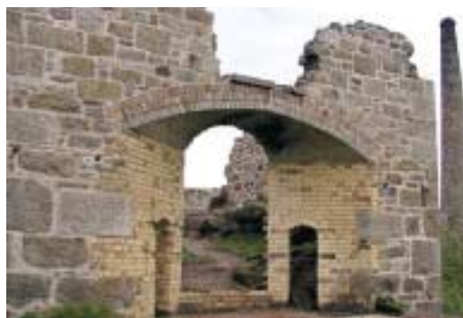
Botallack Mine. The recently (2004) consolidated remains of a Brunton calciner (1906, Scheduled Monument).
