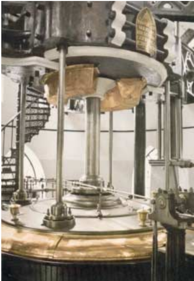
The D F Wouda Steam Pumping Station, Lemmer, Holland (inscribed as a World Heritage Site in 1998). Three Cornish engines were ordered by the Dutch Government in the mid-1840s for the purpose of draining the Haarlem Mere. Two were supplied by Harvey & Co., Hayle, and the other by Perran Foundry, Perran-ar-worthal. The cylinder cover of the Cruquius engine is pictured: with an outer cylinder diameter of 144 inches (3.66m), it is the largest steam engine ever built.
