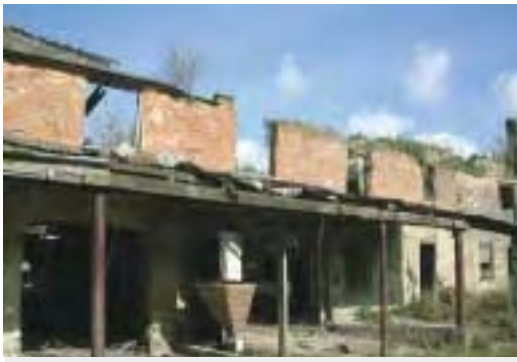
Foundry Farm buildings, Hayle. Part of the Harvey's Foundry complex, these significant industrial buildings await consolidation in Phase II of a regeneration programme led by Penwith District Council.
