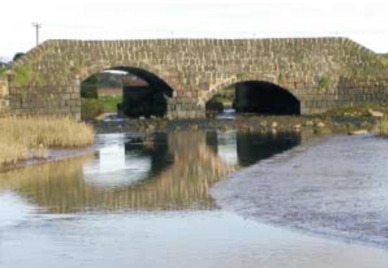
Black Road embankment and Black Bridge (1811, Scheduled Monument). The extensive use of scoria blocks is apparent.
