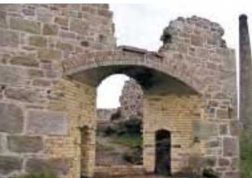
Botallack Mine. The recently (2004) consolidated remains of a Brunton calciner (1906, Scheduled Monument).
