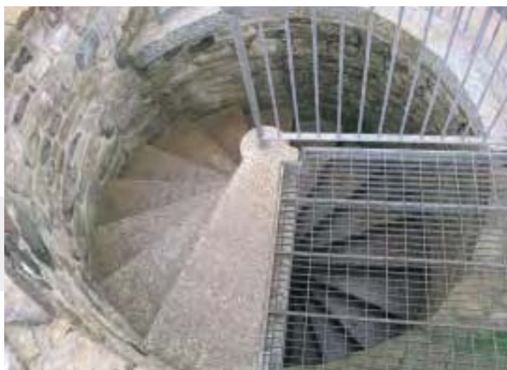
The completed renovation of the Man Engine tunnel and steps at Levant Mine.
