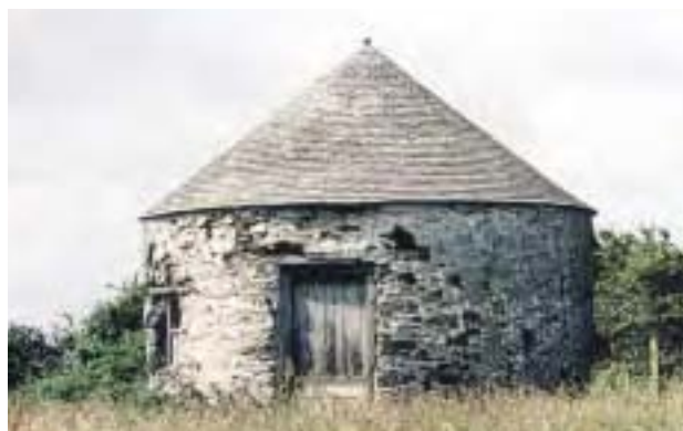
Wheal Clifford powder magazine (Listed Grade II). This example is one of only a few survivals in the nominated Site of this important type of mining structure.
