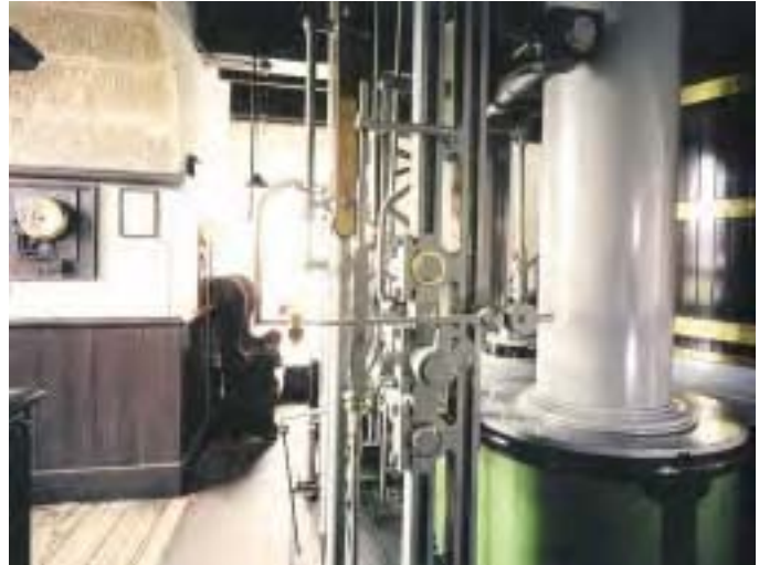
East Pool & Agar Mine (Listed Grade II*). Interior of Taylor's engine house.
