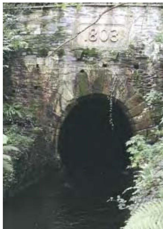
Tavistock Canal tunnel, southern portal (1803, Listed Grade II). Not a single fatal accident occurred during the entire construction of the Tavistock Canal.
