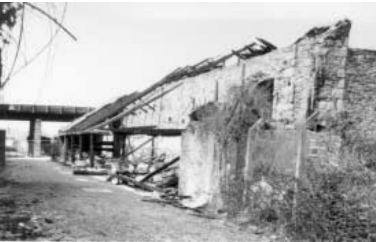
The building at Harveys Foundry, Hayle (A2) is an example of the damage which can be caused by fire, often through arson attack.
