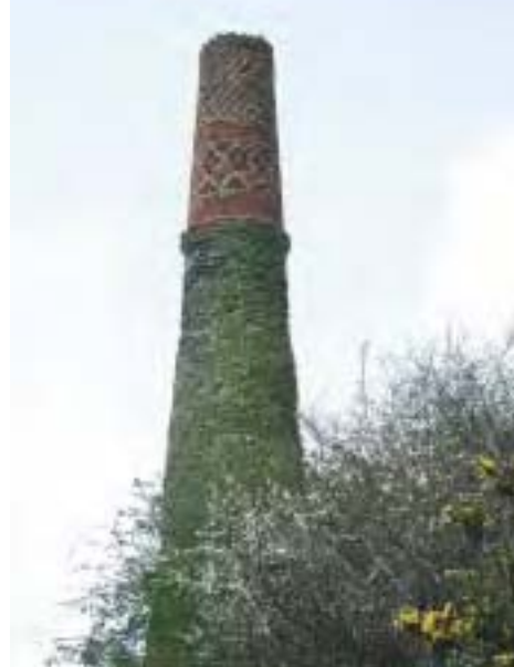
West Wheal Metal (Listed Grade II). Unusual ornamentation in the brickwork of the chimney stack.
