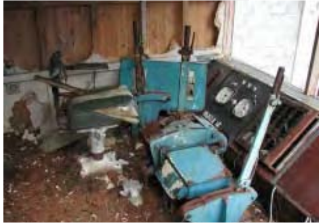
Vandalism within the winder driver's cabin, Robinson's Shaft Complex.
