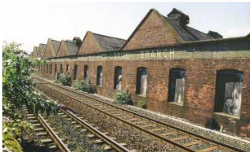
Holman's Rock Drill Works, Camborne (A5). Holman's made a global impact with their rock drills and compressed air mining equipment during the late nineteenth- and early twentieth century. By 1896 there were more than 1,000 Cornish rock drills in use in the Rand gold mines in South Africa. Cornish manufacturers did much to pioneer dust-suppression by delivering a water spray to the drill bit.
