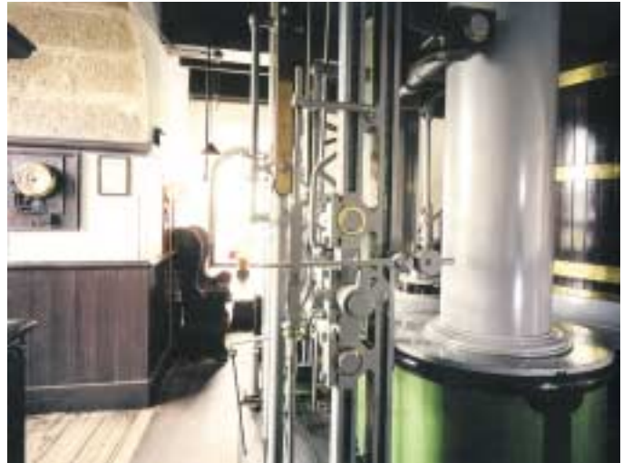
East Pool & Agar Mine (Listed Grade II*). Interior of Taylor's engine house.
