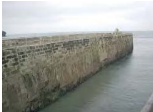
Portreath Harbour breakwater. Coastal defences require regular monitoring and consolidation to maintain their stability.
