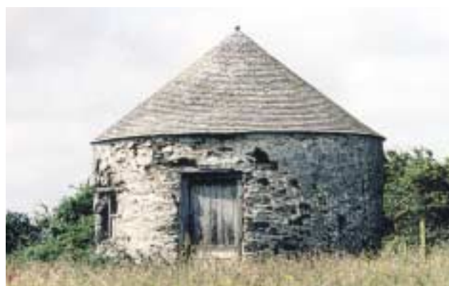
Wheal Clifford powder magazine (Listed Grade II). This example is one of only a few survivals in the nominated Site of this important type of mining structure.
