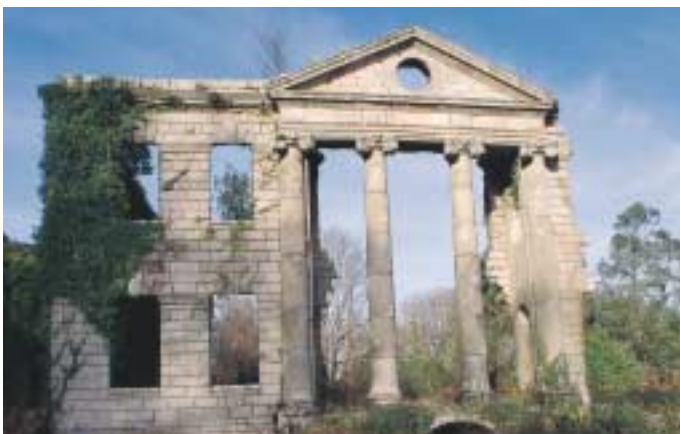
Carclew House (Listed Grade II), Perran-ar-Worthal. Once the home of mining magnate Sir Charles Lemon, Bart. (1784-1868), the house suffered from a disastrous fire in 1934.
