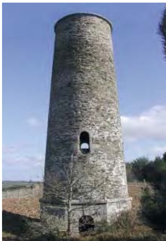
Consolidated Mines. This unusual structure is the base of a clock tower at this mine which produced over 12% of Britain's copper from 1823 to 1835.
