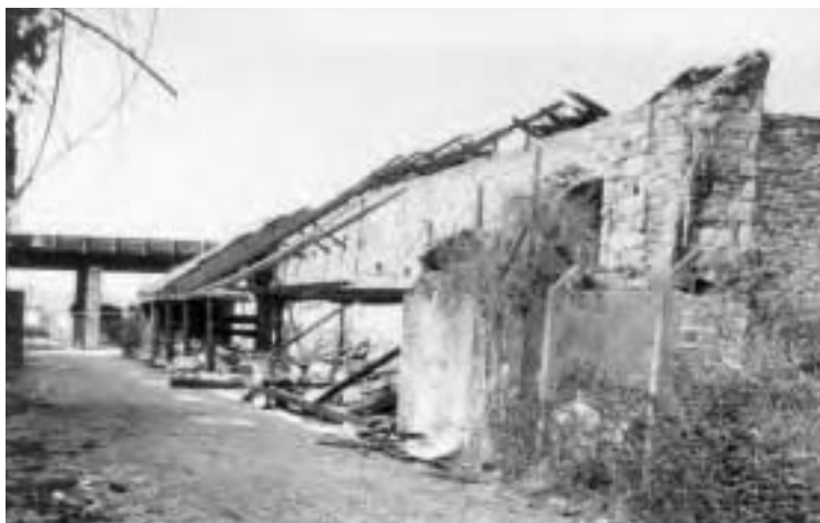
Fire damage at Harvey's Foundry, Hayle.
