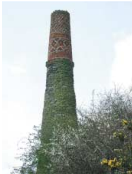
West Wheal Metal (Listed Grade II). Unusual ornamentation in the brickwork of the chimney stack.
