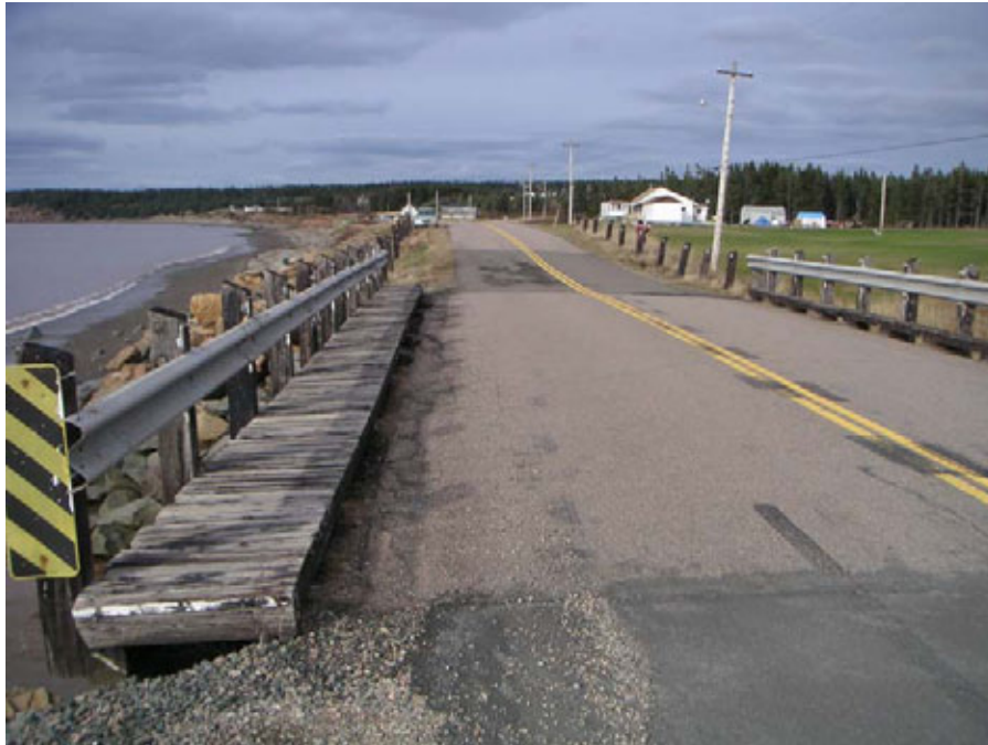
Figure 10 - Lower Cove Bridge looking north showing deteriorated condition
