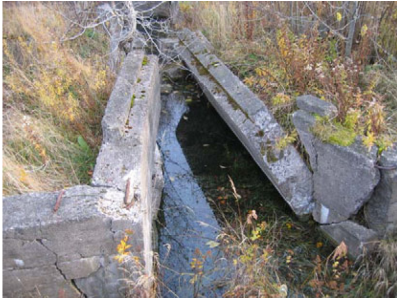
Figure 17 - Collapsing remains of Roundhouse foundation
