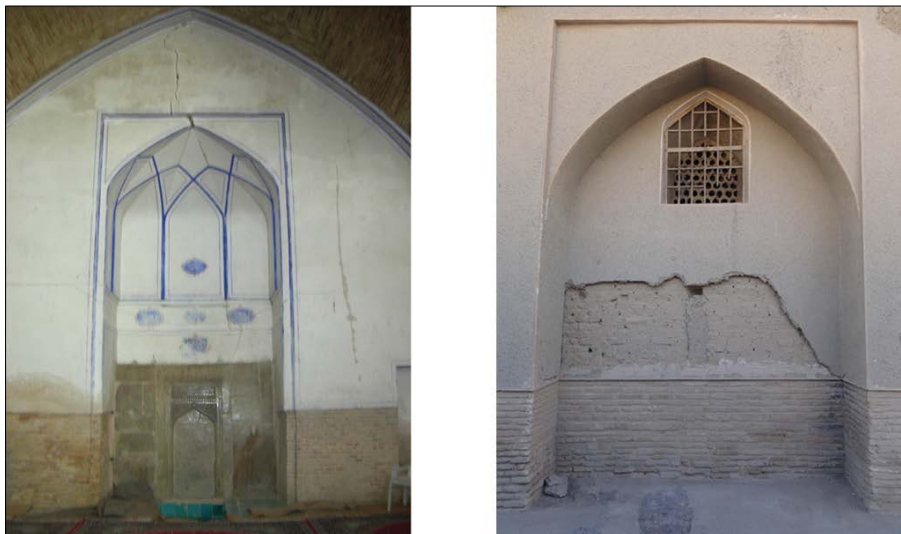
Photo 4-24. Humidity effect on the building (MJIB, Jabal Ameli)
