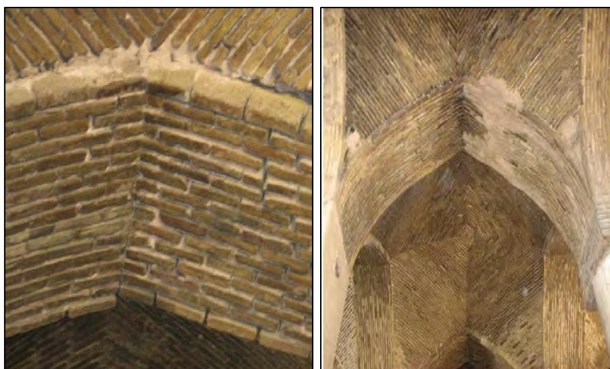
Photo 4-27. Vertical deformation in vaults of Saljuq Shabestan (MJIB, Jabal Ameli)
