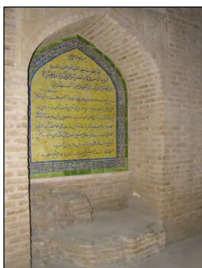
Photo. 5-4. Inscription which contains the information about rebuilding some parts of the Masjed that were destroyed during the 1980s war (MJIB)
