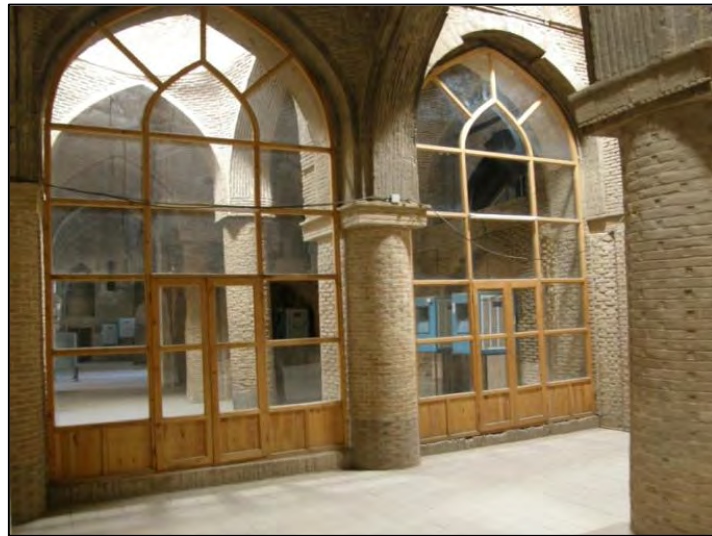
Photo 4-21. Unsuitable temporary cooling and heating system in some parts of the mosque (MJIB)
