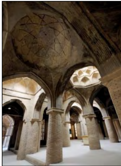
Photo 13. Variety of vaults (Taq-o cheshmehs) in the Seljuq Shabestan (hypostyle part of the mosque)
