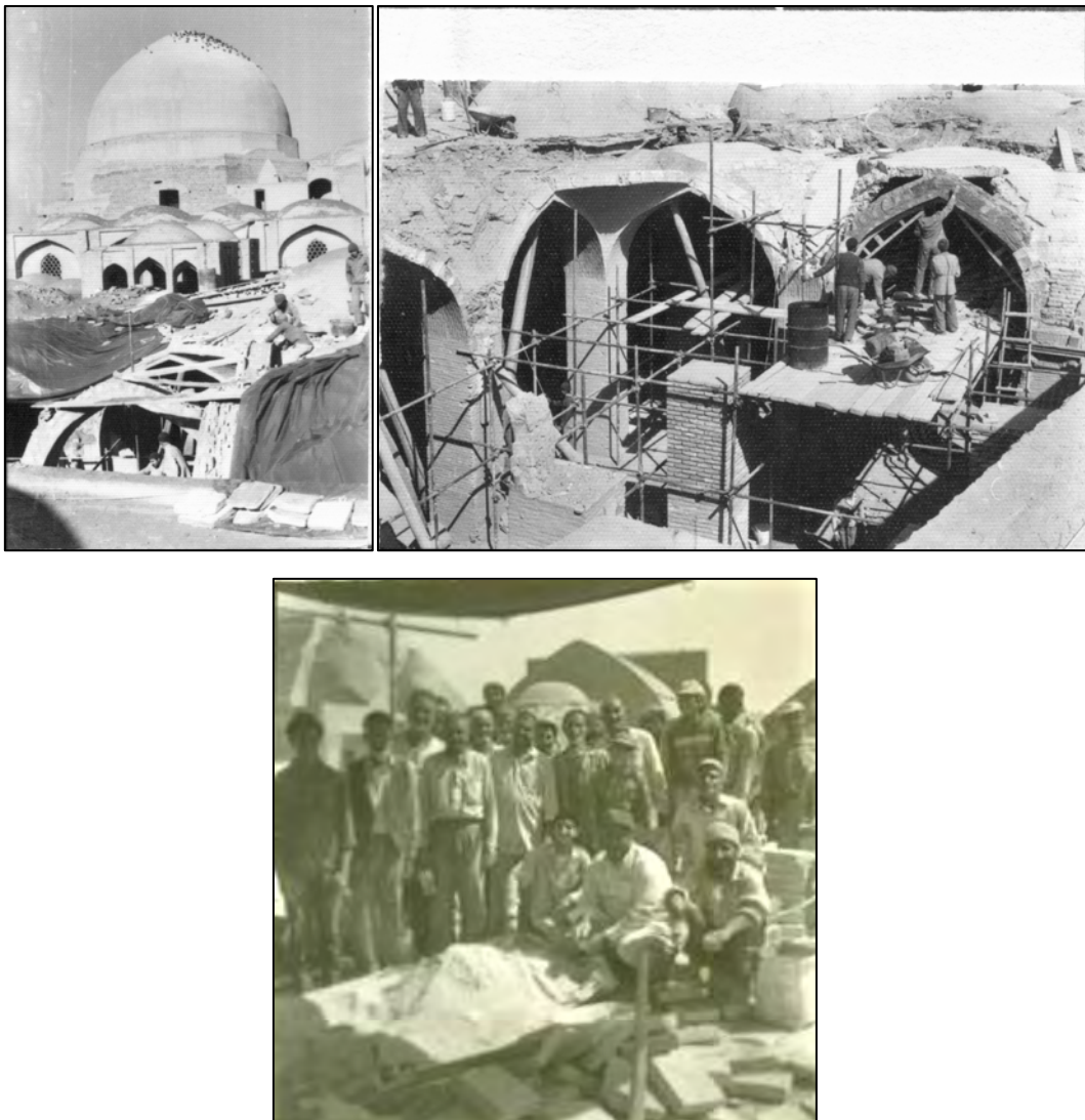
Photo 4-31. Restoring the south east part of Masjed after bomb attack of Iraqi forces in 1985 by ICHO, with the participation of local craftsmen (MJIB, Jabal Ameli)
