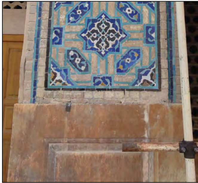
Photo 4-30. Imbalance in plinths (Ezarehs) of the courtyard (MJIB, Jabal Ameli)
