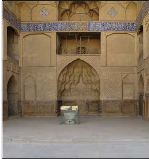
Photo 4-23. Eastern Ayvān affected by rising moisture (MJIB, Jabal Ameli)
