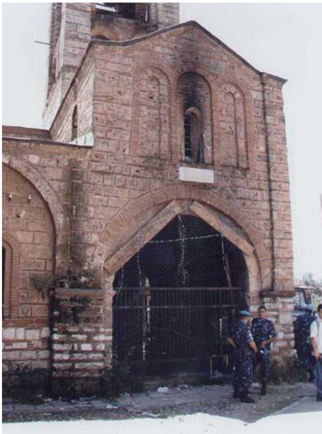
34. Church of the Virgin of Ljeviša, North view of the exonarthex after March 2004 /photo by Dragan Stanojević/
