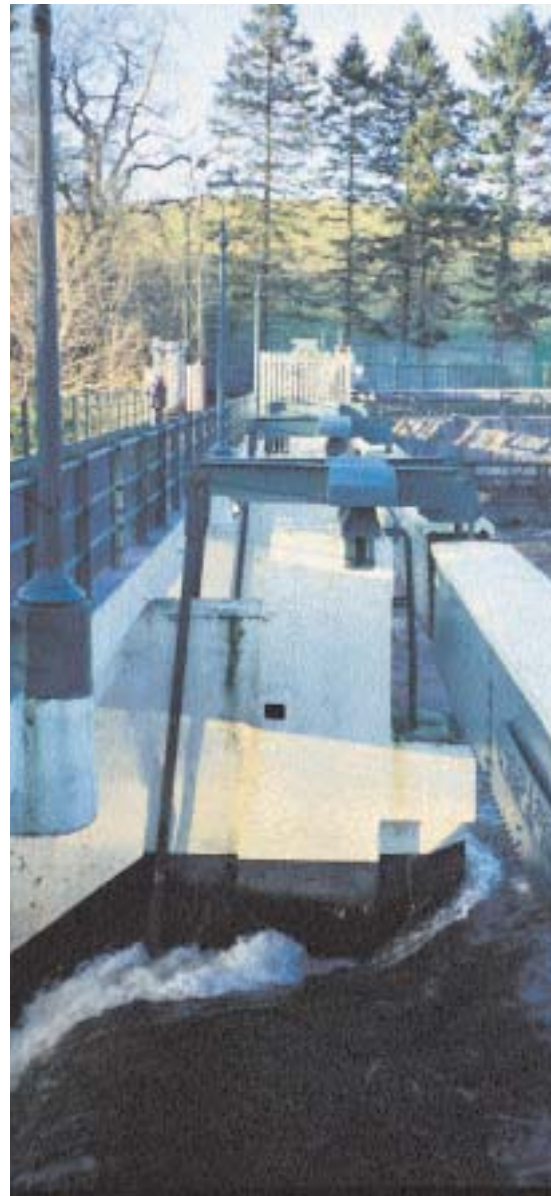
Tilting weir, Bonnington
