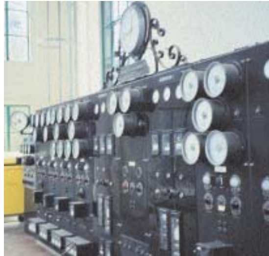
The old switch gear, February 2000
