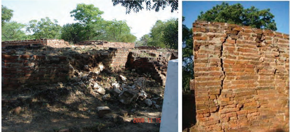
INADEQUATE REPAIR WORK USING CEMENT UNDERTAKEN IN THE PAST AT KKG-3 AND KKG-2 (BEIKTHANO)
