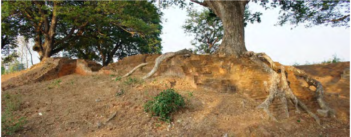
MONUMENT SHOWING THE PENETRATION OF TREE ROOTS IN TO THE GATE (SRI KSETRA)
