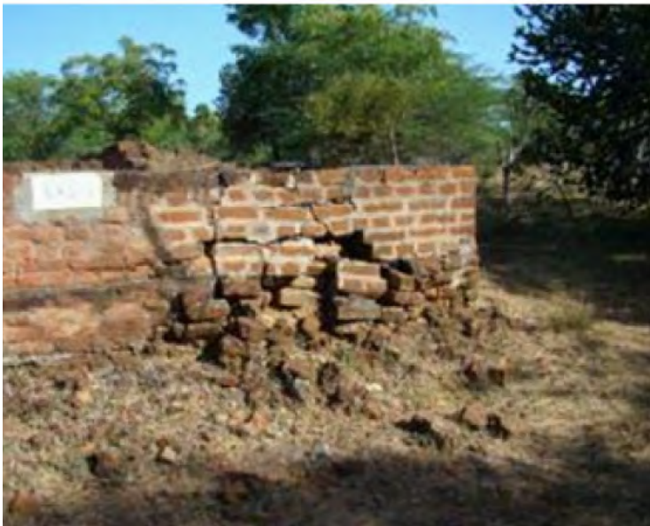
KKG4 (2009) DETERIORATION OF ORIGINAL BRICKS DUE TO USE OF CEMENT AND MODERN BRICKS (BEIKTHANO)
