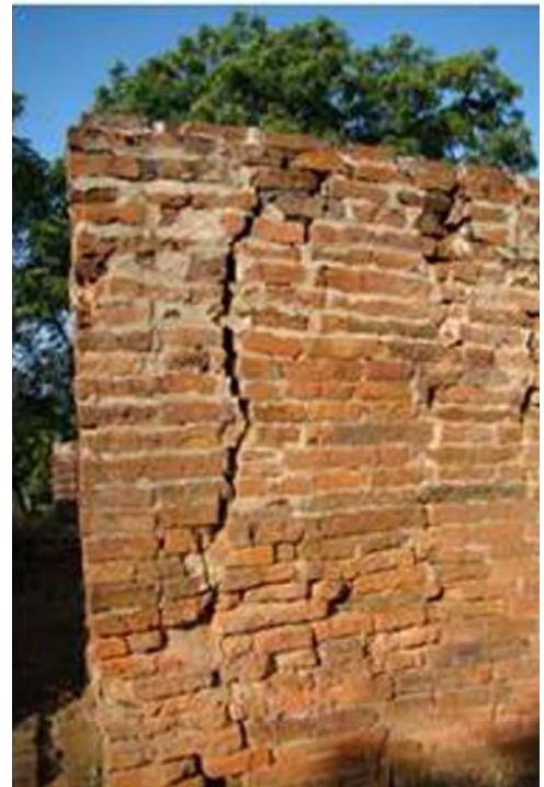
CRACKED BRICKWORK DUE TO OVERLOADING AT KKG-2 (BEIKTHANO)
