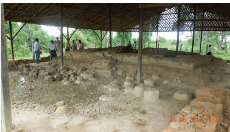
MEMORIAL HALL BTO-28 WITH BURIAL URNS WHERE SHELTER HAS PROVIDED ONLY PARTIAL PROTECTION (BEIKTHANO)
