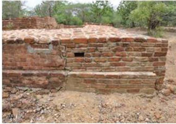
MEMORIAL HALL KKG-4 WITH INADEQUATE CONSERVATION OF BRICKWORK (BEIKTHANO)
