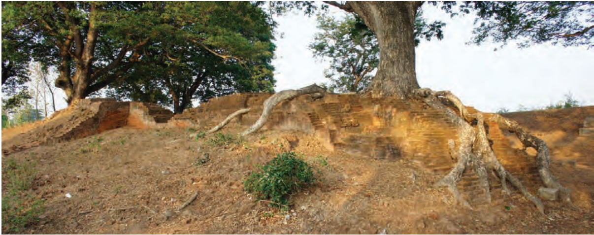
PENETRATION OF TREE ROOTS INTO ANCIENT STRUCTURE (SRI KSETRA)
