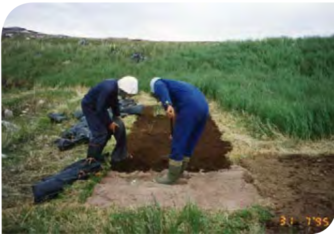
Figure 4.4 Stabilization of excavated area at the Saddle Island West site. Parks Canada
