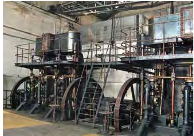
Figure 8: Trieste, Old Port, hydraulic power plant, machinery room
