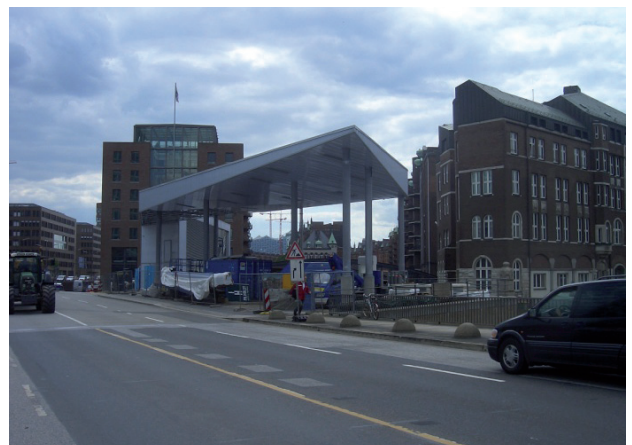
Fig. 65: View from Oberbaumbrücke to the Speicherstadt as it is at present, blocked by the construction of a new hydrogen filling station
