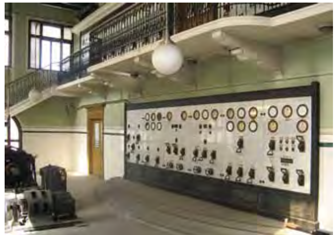
Figure 14: Trieste, Old Port, power plant
