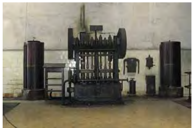
Figure 10: Trieste, Old Port, hydraulic power plant, (1890) auxiliary machine Breitfeld & Danek – Karolinental – Prag
