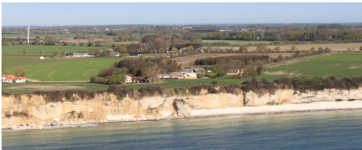
Figure 13. An additional example of cliff-fall from the inner part of Lille Hedding Vig (Loc. 4 in fig. 1). The cliff-fall is seen just below the yellow house, and its dimension of 1200 m 3 corresponds well with the general magnitude of cliff-falls.
