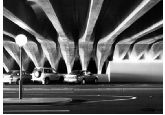
41. Timber partition obscuring dramatic descent of folded beams in vehicle concourse. JSK photograph 98.8.3.
