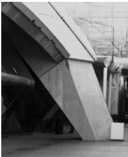
63. 1993 photograph of broken edge tiles before replacement and pedestal feet wearing their new socks. JSK photograph 93.5.27.
