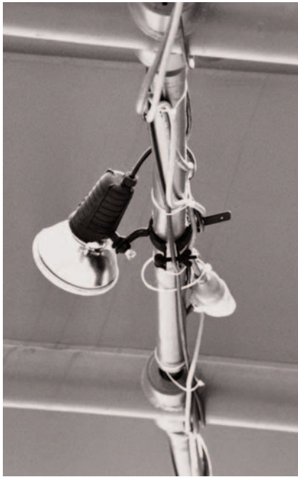
51. Supplementary lighting and conduits between the mullions above the north foyer of the Concert Hall. JSK photograph 93.6.5.
