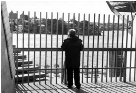
37. 'Safety' pickets added to the rail at the northern lip of the podium. JSK photograph July 2002.
