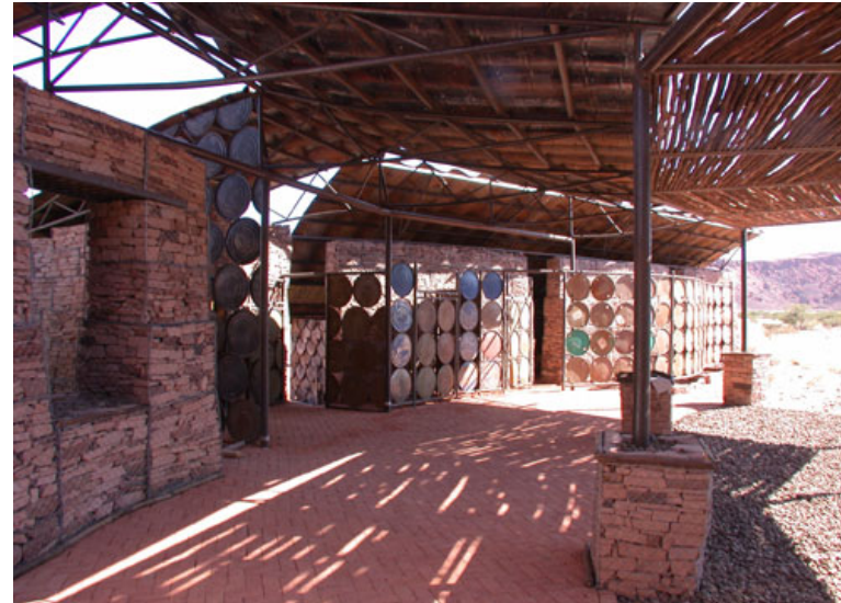
Visitor Centre under construction, showing combination of building materials and techniques (Nina Maritz Architects)
