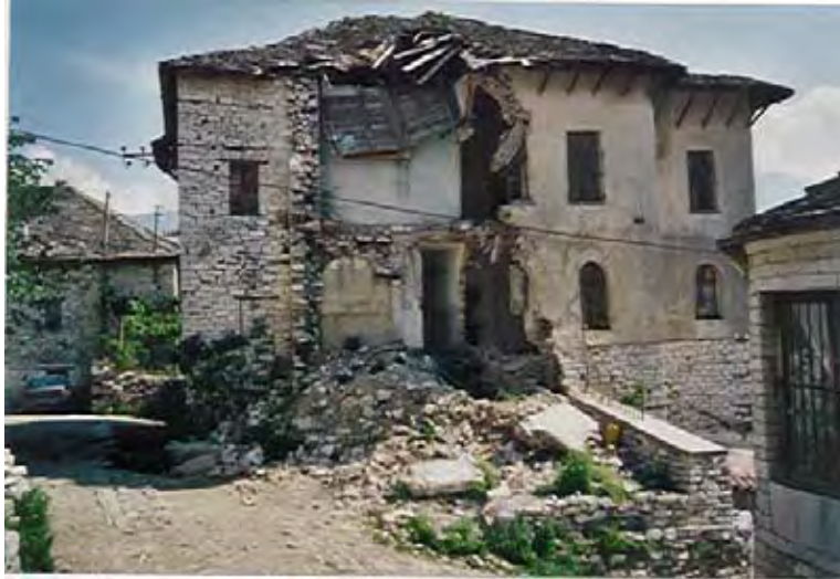
Fig. 34 – Bazaar building in a ruinous state
