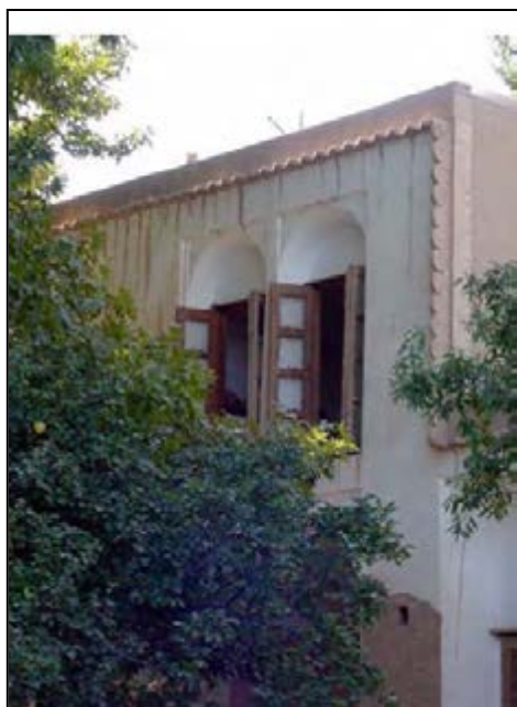
Fig.4-103. Affect of falling damp on the façade (Base of the Persian Garden, Yazd)
