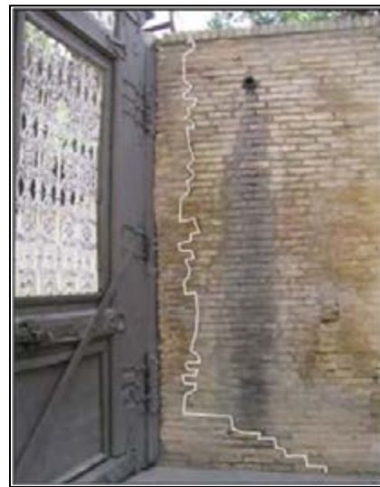
Fig.4-77. Affect of falling damp in Northern entrance (Fazlinezhad)
