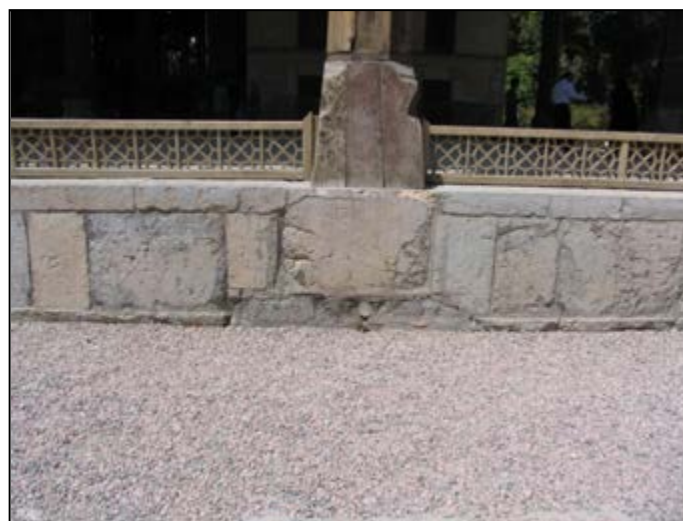
Fig.4-78. Erosion of Stone plinths because of environmental factors (Fazlinezhad)
