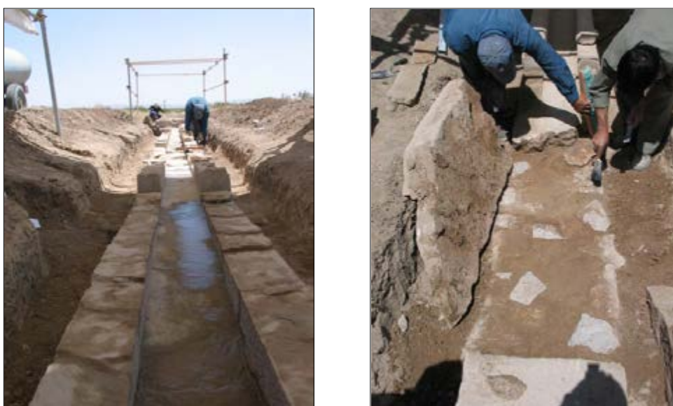
Fig.4-6. Restoration phases of Bagh-e Shahi fountains: cleansing and brushing pieces, patching, steel inserting and grouting (Archives of Research Foundation of Parse-Pasargadae )
