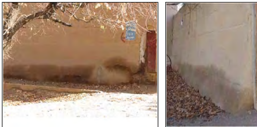
Fig.4-102. Rising damp in the enclosure of the garden (Base of the Persian Garden, Yazd)
