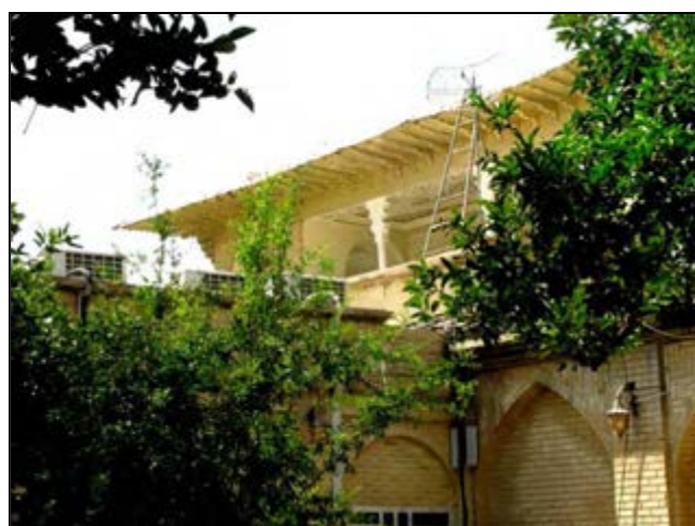
Fig-4-68.Electrical utilities on the Sharbatkhaneh pavilion’ facade (s. malekpur)
