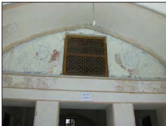
Fig.4-80. The main facade of Safavid Kushk in front of the main facade of the garden, decay in chalk decoration (Khoshnood)
