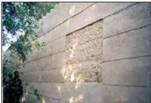
Fig.4-51. After restoring the mud wall surrounding the garden (The Base of Persian Garden, Yazd)
