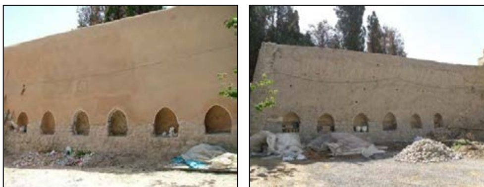
Fig.4-19.Restoring of the walls of the garden (The Base of Persian Garden, Isfahan)
