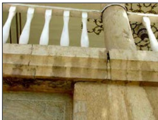
Fig.4-72.Erosion in Main Ivan (S.Malekpur)
