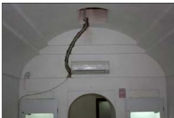
Fig.4-108. Heating and cooling utilities in the building (S. Kelayeh)
