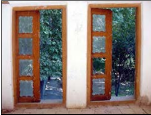
Fig.4-105.Deterioration of wood works (Base of the Persian Garden, Yazd)
