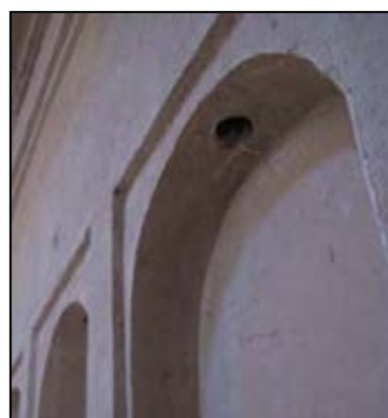
Fig.4-101.Unsuitable electrical utilities in the building (Base of the Persian Garden, Yazd)
