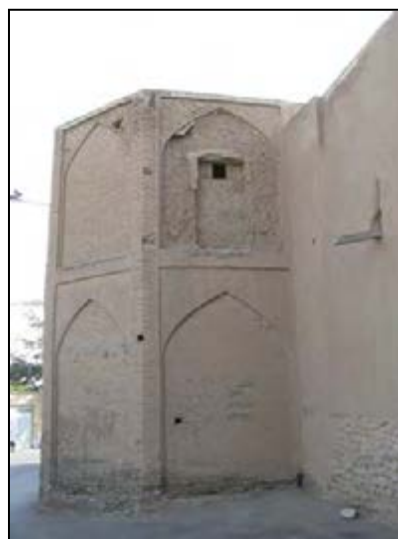
Fig.4-82. the entry behind the museum of Bagh-e Fin , deterioration due to rising damp (Khoshnood)
