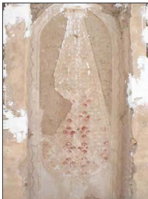
Fig 4-97. Deterioration of winter pavilion decoration (Qajari)
