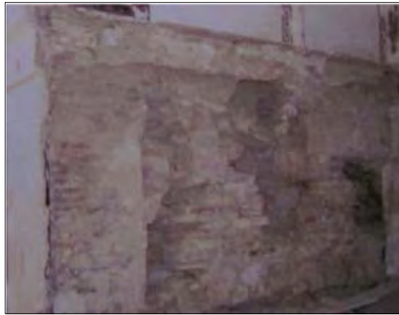
Fig . 3-109. Qajars basin house niches before restoration (Kashan ICHHTO Archives)
