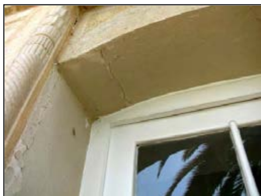
Fig.4-71.Erosion in the Main Ivan (S.Malekpur)
