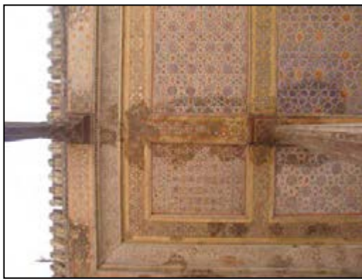
Fig.4-76. The trace of the falling damp on the Kushk ceiling (Fazlinezhad)
