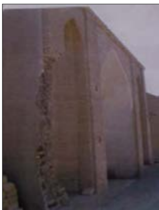
Fig. 3-130. Before restoration (Kashan ICHHTO Archives)
