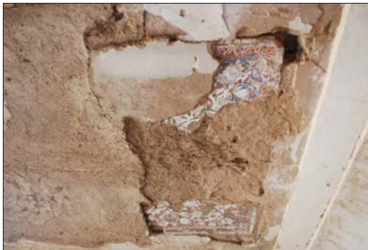
Fig.4-98.Kahgel coat eroded because of termite (Asadi)
