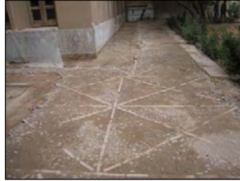
Fig.4-106.Affect of falling damp on the stone pavements (Base of the Persian Garden, Yazd)
