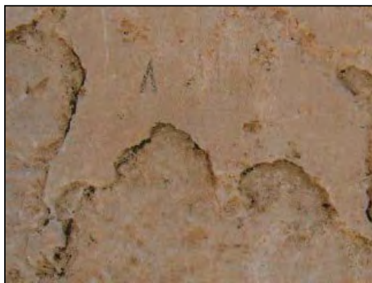
Fig.4-60.Flaking of stones, Palace P (Parse-Pasargadae Research Foundation Archives)
