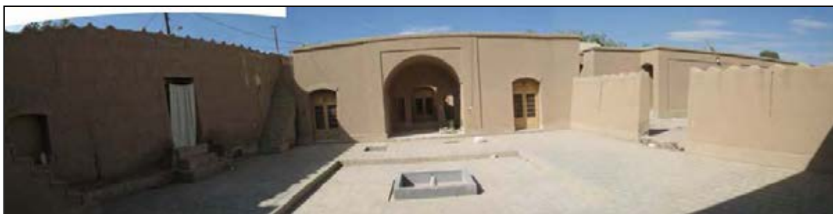
Fig.4-49.T pavilion after repair and maintenance activities (The Base of Persian Garden, Yazd)
