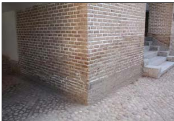
Fig.4-109. The affect of rising damp on the building (S. Kelayeh)
