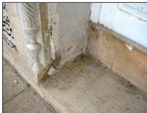
Fig.4-70.rising damp in external wall of the main pavilion (S.Malekpur)
