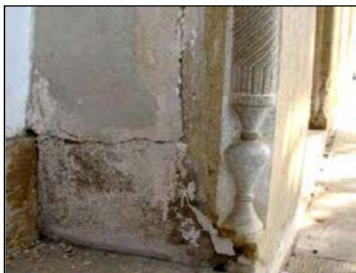
Fig.4-69.rising damp in external wall of the main pavilion (S.Malekpur)
