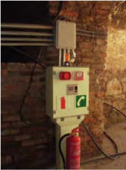
001 089 INTERCOM SYSTEM IN GALLERIES. EXAMPLE.
