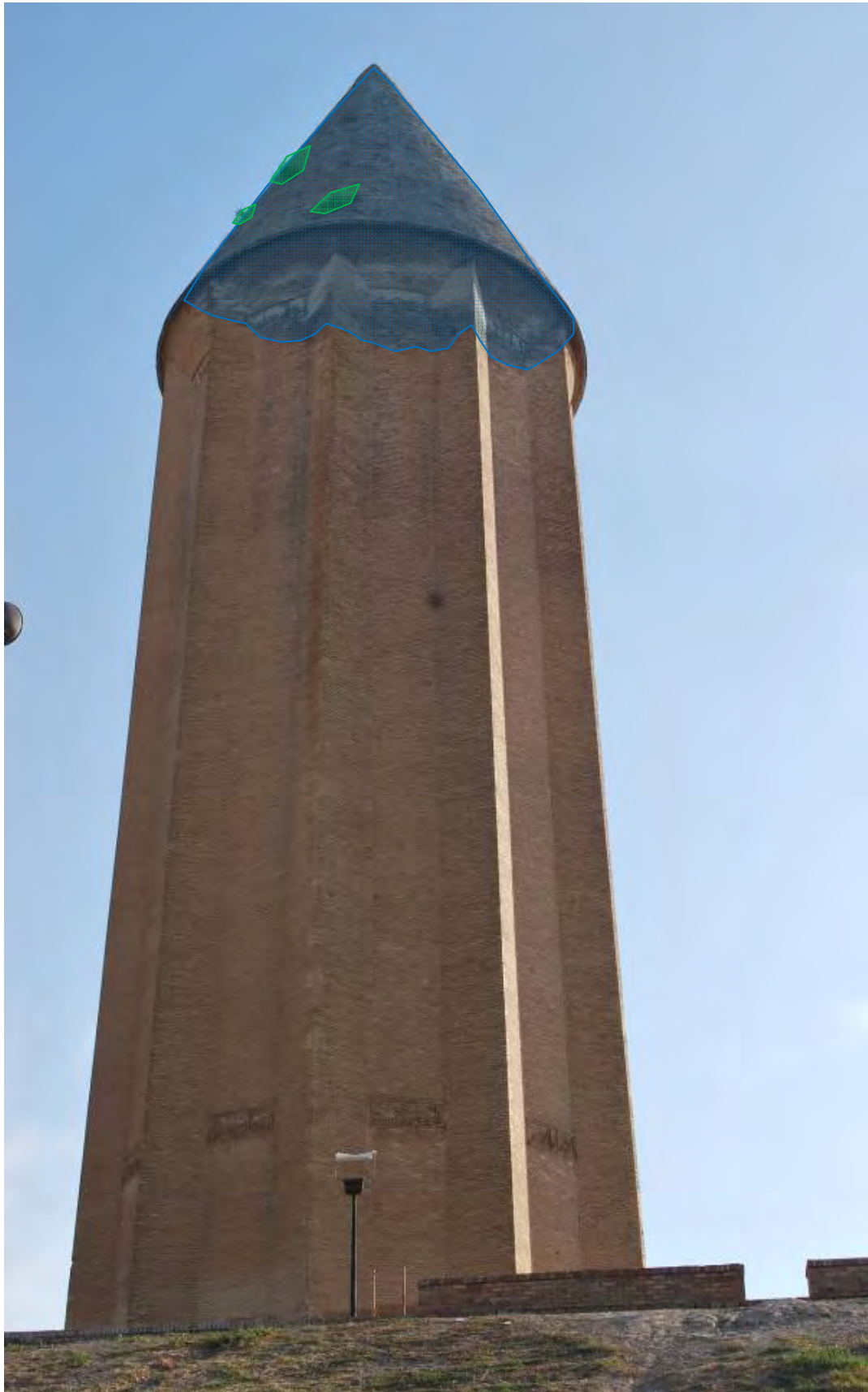
Figure .4. -Ascending moisture on the top of the roof
