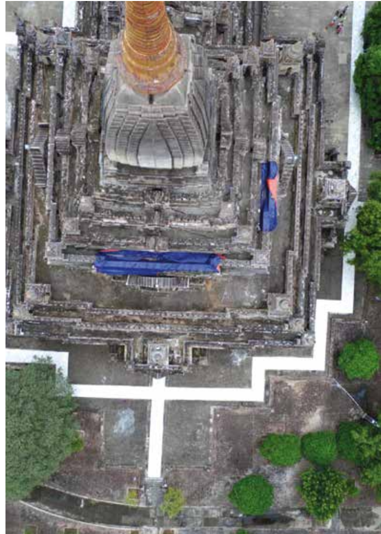
▲ A DRONE IMAGE OF A DAMAGED MONUMENT IN BAGAN © Davide Mezzino/Ross Davison
