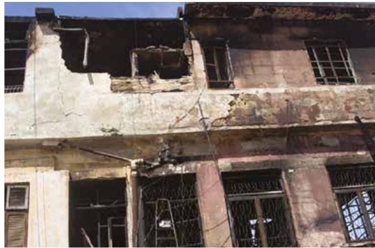
▲ DAMAGED BUILDINGS IN DAMASCUS
