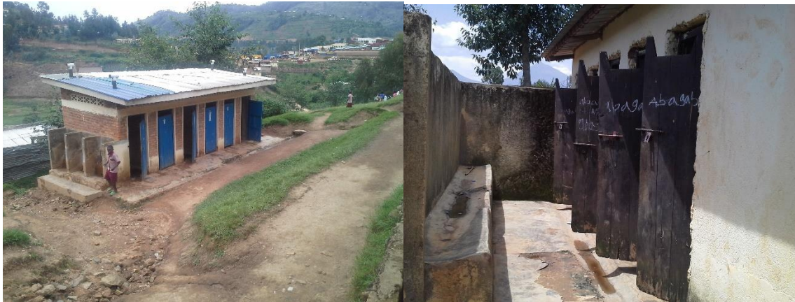
Figure 4: Poor maintained toilets in Kirambo Primary School, Burera District and Musero Primary School, Musanze District
