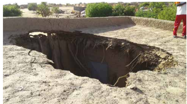
▲ THE PARTIAL COLLAPSE OF THE ROOF OF THE PRAYING ROOM AT THE TOMB OF ASKIA (MALI) © UNESCO/S. Diallo
