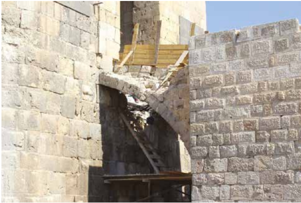
▲ EMERGENCY CONSOLIDATION WORKS ON THE ENTRANCE AND BRIDGE OF THE CITADEL OF ALEPPO (SYRIAN ARAB REPUBLIC) © UNESCO/DGAM
