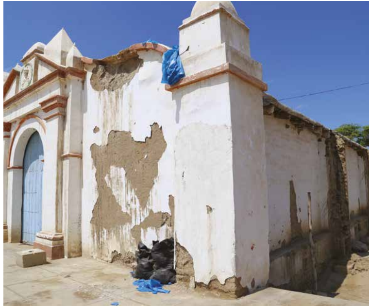
▲ DAMAGED CHURCH IN LAMBAYEQUE (PERU) © UNESCO
