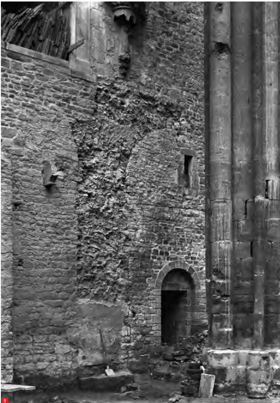
Minden, Cathedral: break-off traces of the wall projection and the barrel vault attached above it between the northern isle of the central room and the northern isle of the westwork in 1950
