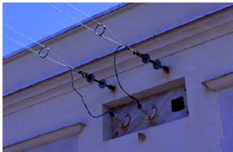
Exit of feeder line from transmitter building, 2000
