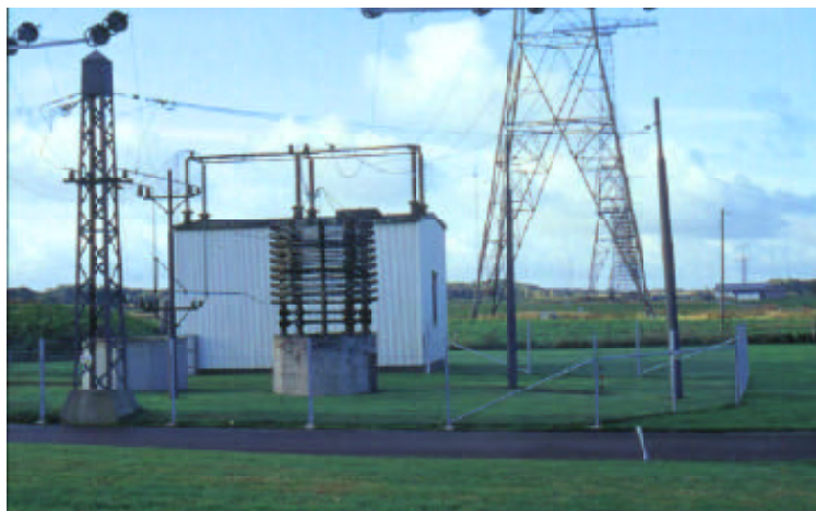
Feeding end of the antenna, showing tuning coil and ice-melting transformer house, 2001
