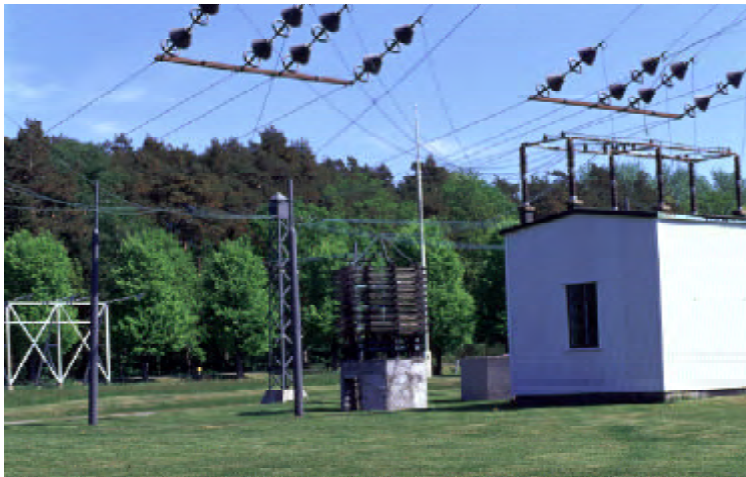
Feeding end of the antenna, showing tuning coil and ice-melting transformer house, 2000
