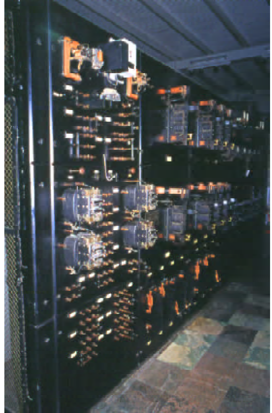
Relay panel of the keying system, showing high-power keying relays, 2001 Photo: Bengt Spade
