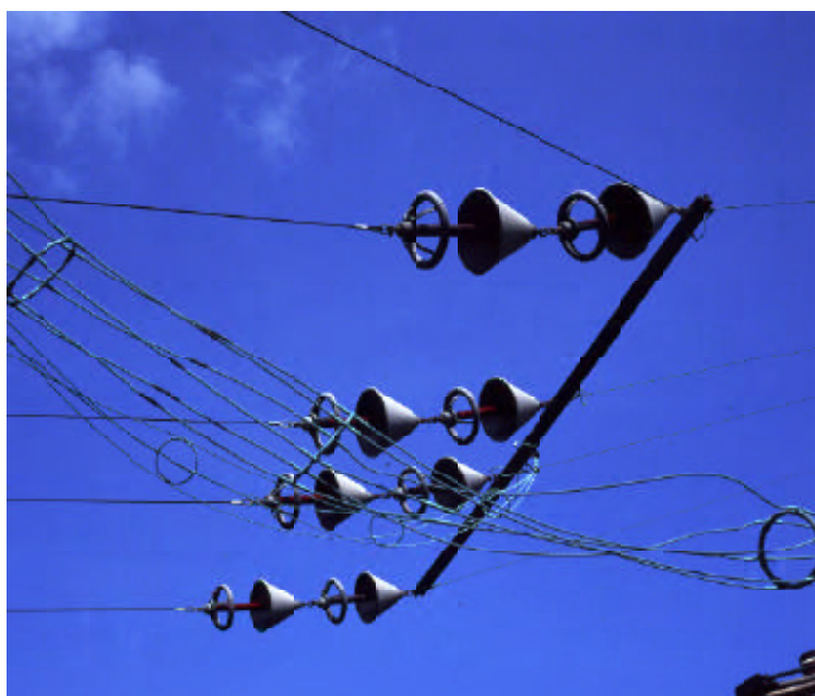
Detail of insulators, 2000
