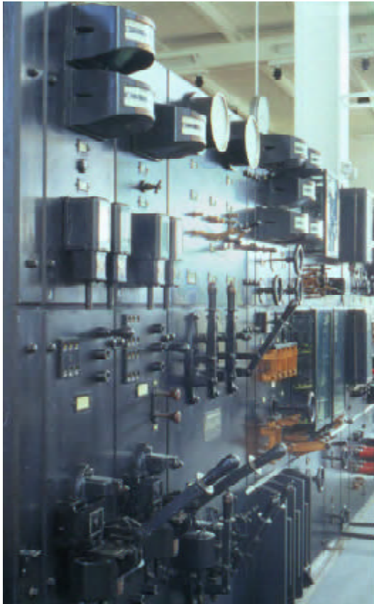
Switchboard, 2001 Photo: Bengt Spade
