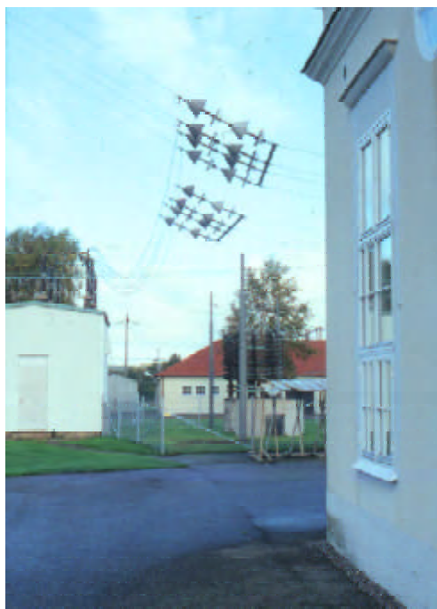
Tuning coil and insulators, 2001.
