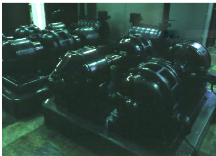
Motor generators, 500V, and 125/250V, 2001
