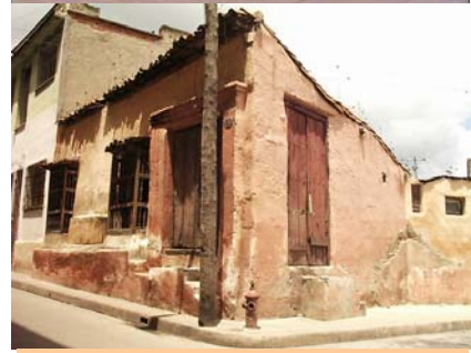
Some very ancient houses keep good conditions, but others need to be repaired.
