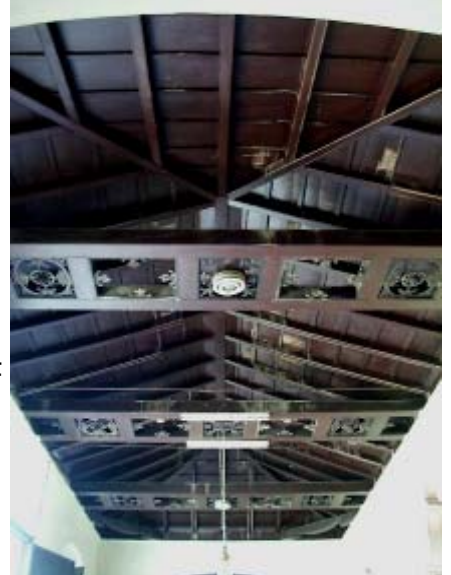
The Mudejar framework of the roofs with braces, angle braces and bowses
