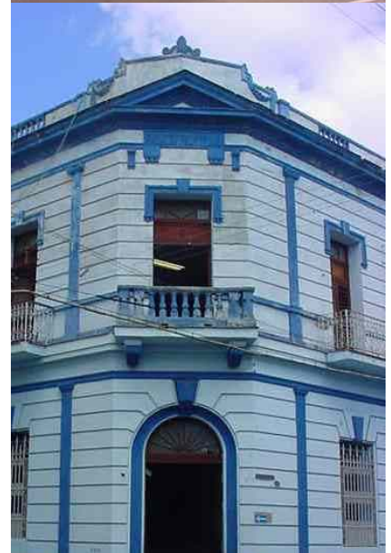
The current civil repertoire is manifested through meritorious exponents of architectural value in which can be identified clearly the different stylistic influences.
