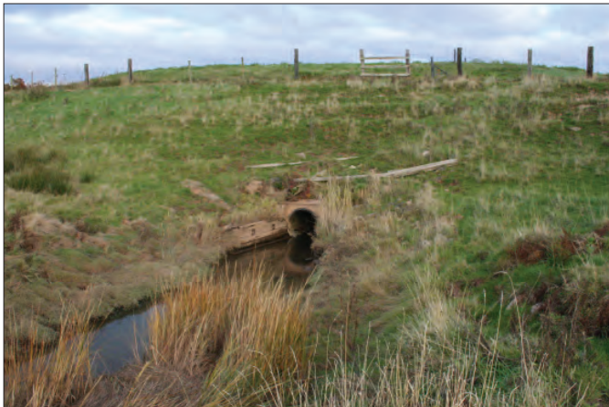
3–16 Five aboiteaux drain the dykelands on the nominated property.
