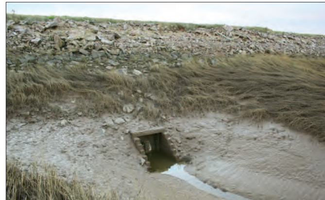
3–9 The dykeland at the Landscape of Grand Pré continues to be solely used for agriculture. It also continues to use a simple system of drainage, including the aboteau shown here, to drain the dykelands.
