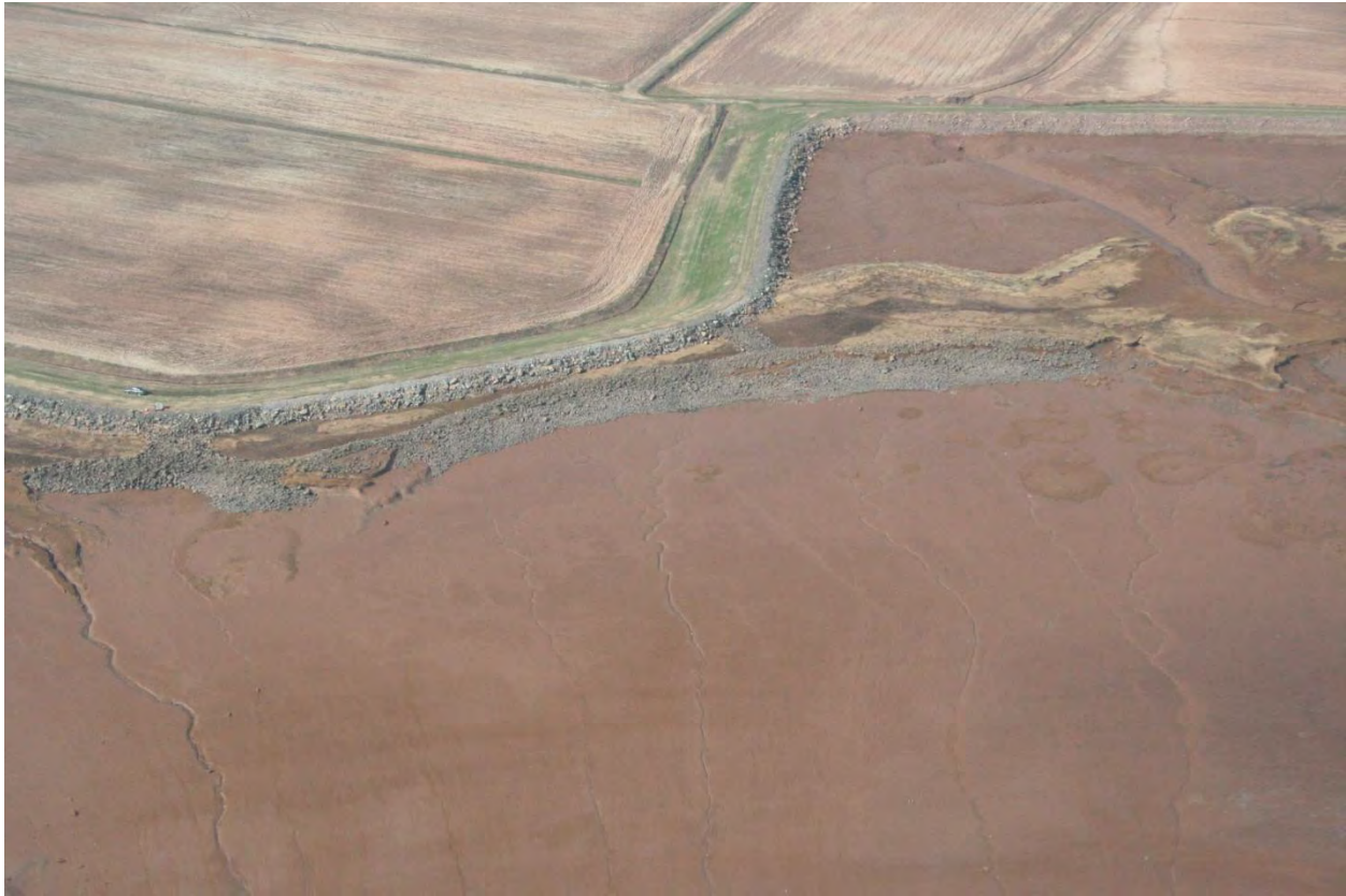
Figure 13: Coastal erosion is a constant pressure on the dykes. Above is a picture of the east facing dykes at extreme low tide. Top right corner: remnants of the salt marsh. In the middle: rock facing on the dykes and breakwater. Both have been weakened by the constant tidal pressure.
