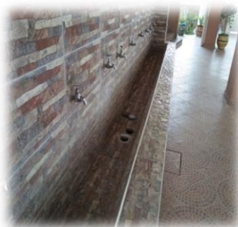
Water conservation by harvesting used water
