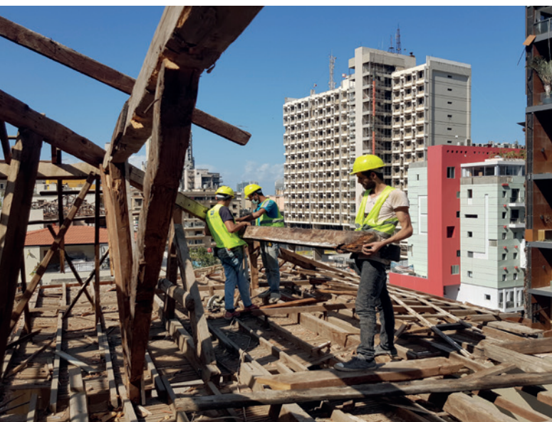
▲ PITCHED ROOF CLEANING AND CONSOLIDATION WORKS UNDERWAY IN BEIRUT (LEBANON) IN ORDER TO SECURE THE BUILDING BEFORE PROCEEDING WITH WOOD RESHAPING © UNESCO
