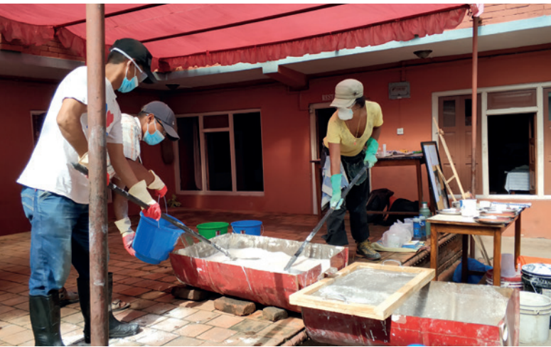
▲ TRAINING ON LIME MORTAR PREPARATION TO IMPROVE THE QUALITY OF MASONRY STRUCTURE IN THE RESTORATION AND REBUILDING OF CULTURAL HERITAGE © UNESCO
