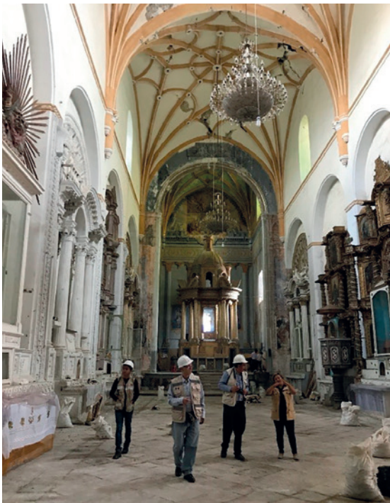
▲ STRUCTURAL REINFORCEMENT OF THE MOST ENDANGERED PARTS OR BUILDING COMPONENTS, AND DEVELOPMENT OF GUIDELINES FOR THE PREPARATION OF A RESTORATION PLAN OF THE STRUCTURE © UNESCO / Inti Muñoz
