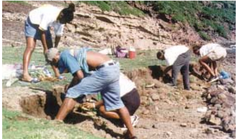
Students building stone barriers and planting cacti to prevent soil erosion, Park Bay, Bequia, St Vincent and the Grenadines. 1997.
