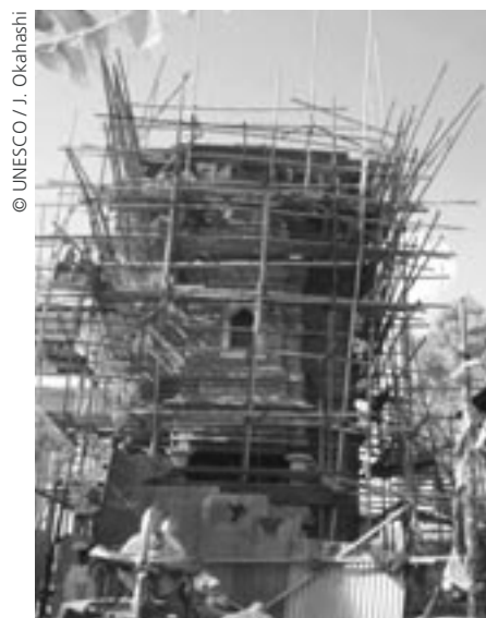
Restoration work of the Prattapur shrine in Swayambunath, Kathmandu Valley, Nepal, financed by national and international funding
