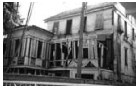
Chess Hall in Georgetown (Guyana): situation in 2002, it collapsed soon after and has disappeared from Georgetown's historic streetscape
