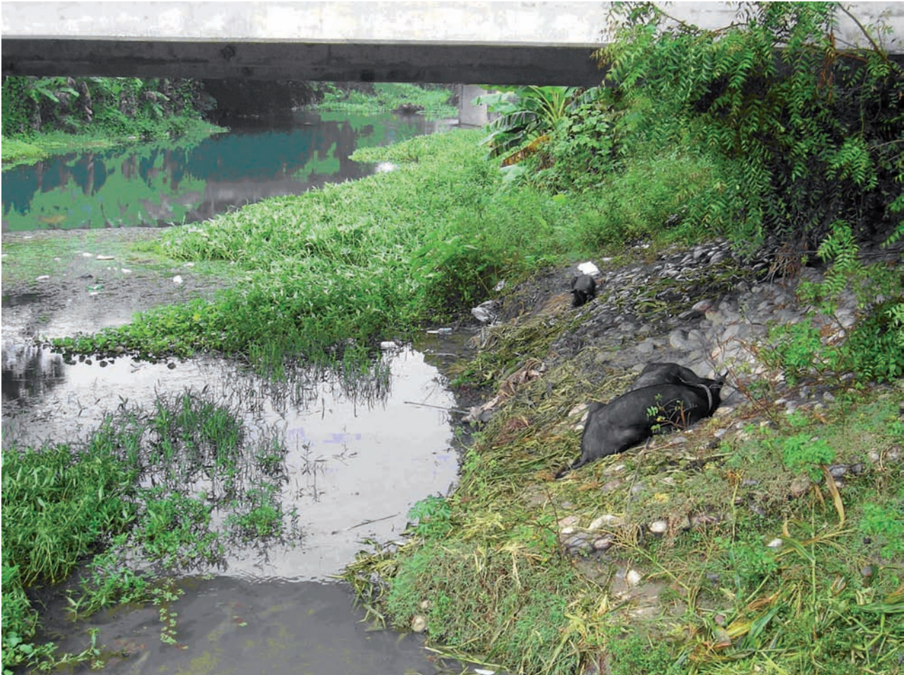
Photograph 1: Bridge over The Islet River at the eastern entry of Cayes (no. 4): water loaded with organic and sediment material clogged by aquatic plants and frequented by domestic animals.
