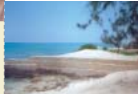
Groynes result in sand build-up on one side, but erosion on the other side, Grand Turk, 1997
