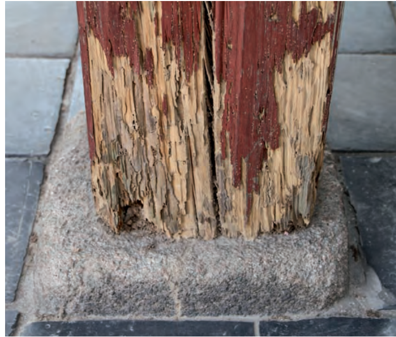
Damage on wooden structures caused by termites.
