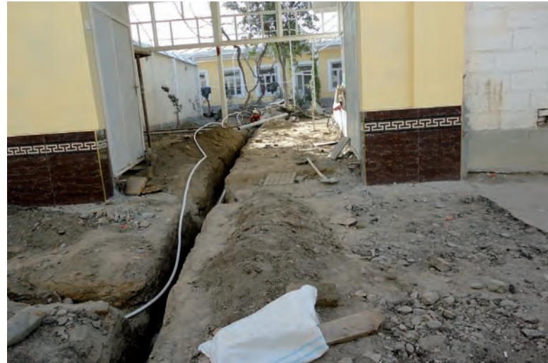
Basic services are a necessity but care should be taken to ensure minimum impact on properties.
