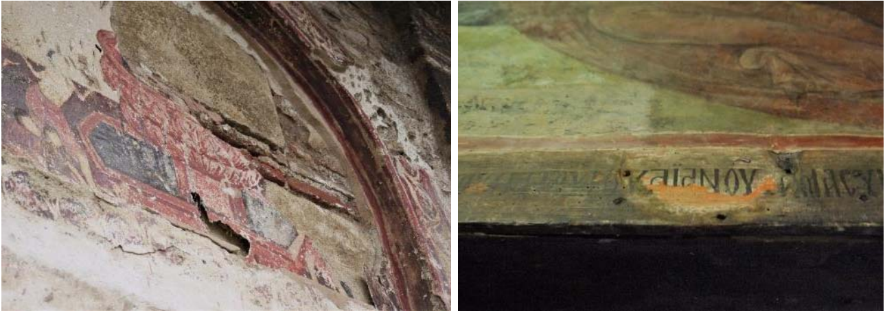
Decorative features and architectural elements both within and without the Byzantine churches showed the need for conservation interventions to halt decay. (© Sarah Court/ICOMOS)
