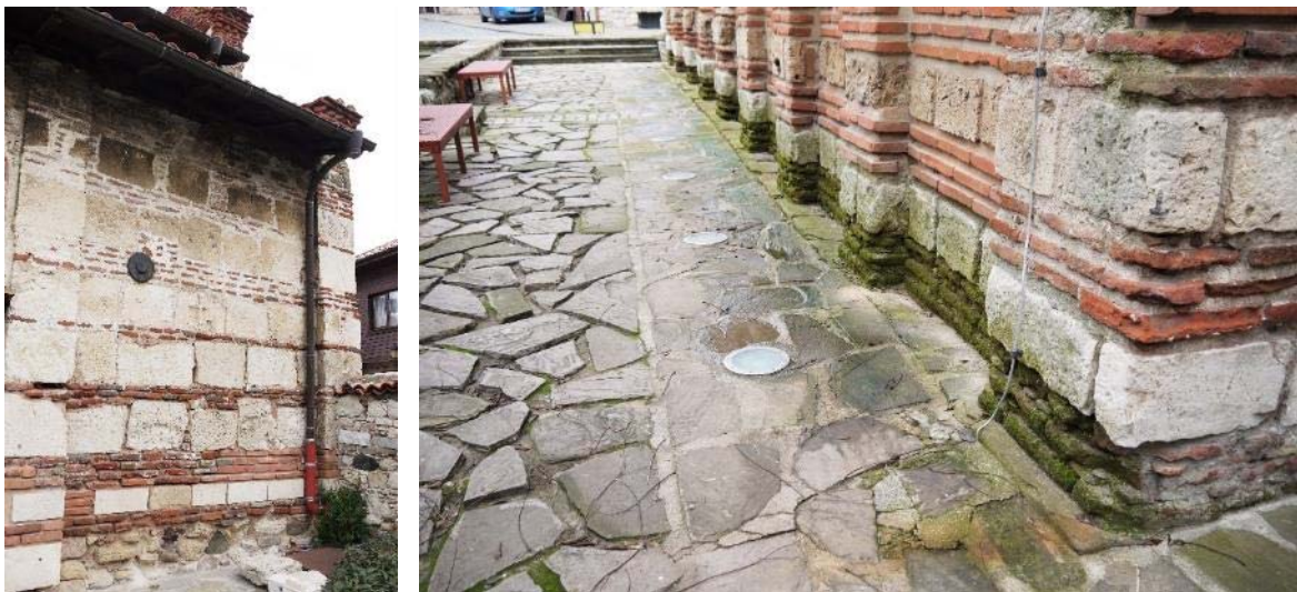
Rainwater management needs to be addressed at more than one church, as there are signs that rising damp is a cause of decay. Left: the Church of St Stephen; right: the Church of St Paraskeva. (© Sarah Court/ICOMOS)
