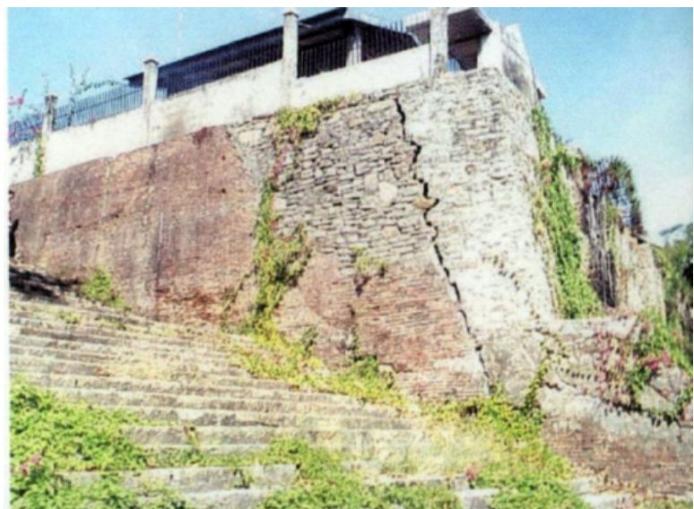
Cracks in the retaining wall of Sta Maria Church, Ilocos Sur
