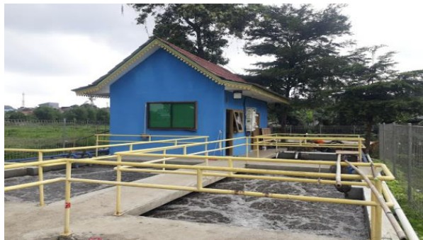
Central of wastewater Treatment (interceptor system)
